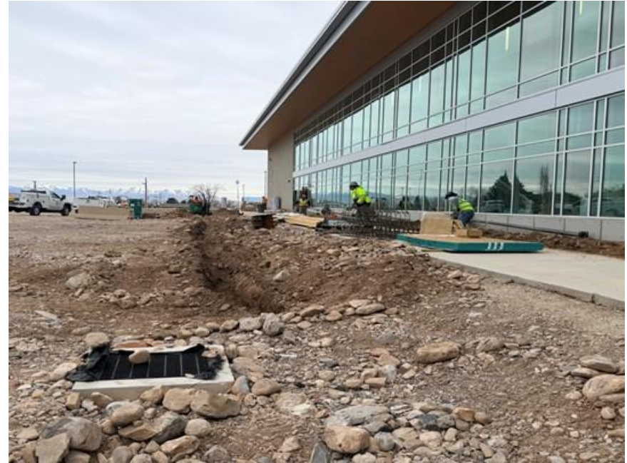
Lighting installation around Performing Arts
