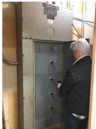
Figure 21 Distribution Panel located in Cafeteria/Gymnasium Area
