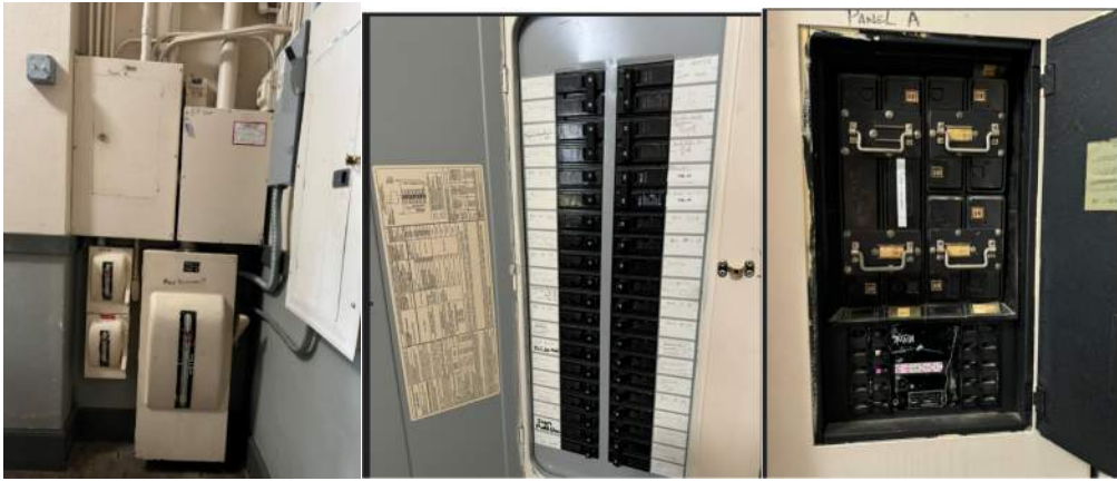
Figure 18 District Office Panels and Disconnects
