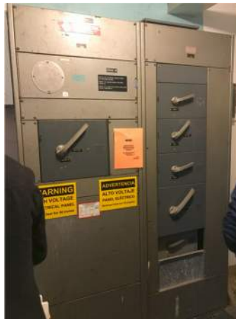
Figure 14 Existing Electrical Service #2
