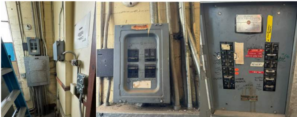
Figure 20 Load centers in existing Shop Building
