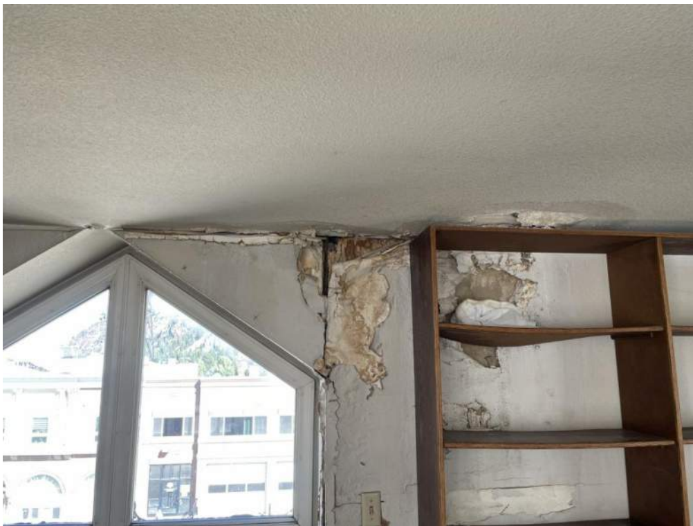
Figure 8- Damage at third floor bay window.
