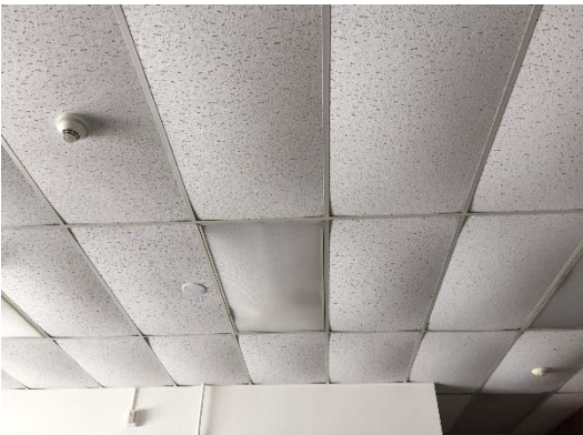
Figure 6: Typical sagging ceiling
