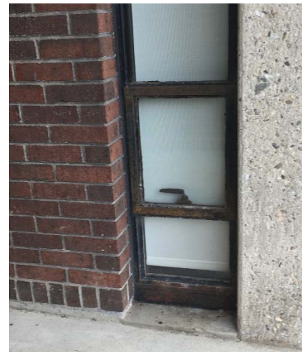
Figure 8: Original Window condition
