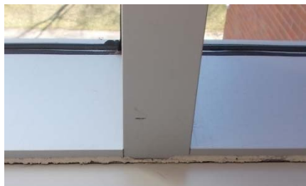
Figure 6: Window caulk cracking
