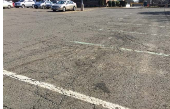
Figure 3: Typical parking lot cracks at front
