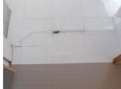
Figure 5: VCT cracking near stair
