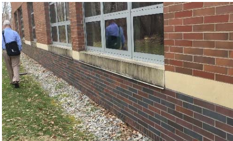
Figure 6: Window sill condition
