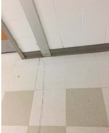
Figure 4: Cracked VCT where expansion joint is needed
