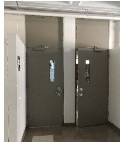
Figure 5: Original classroom doors without required push pull clearance
