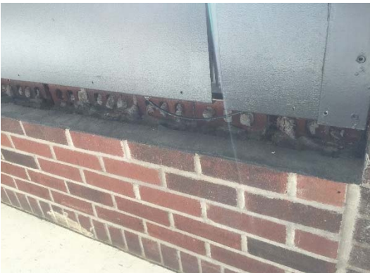
Figure 5: Below window wall missing brick course
