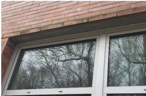
Figure 7: Window head condition
