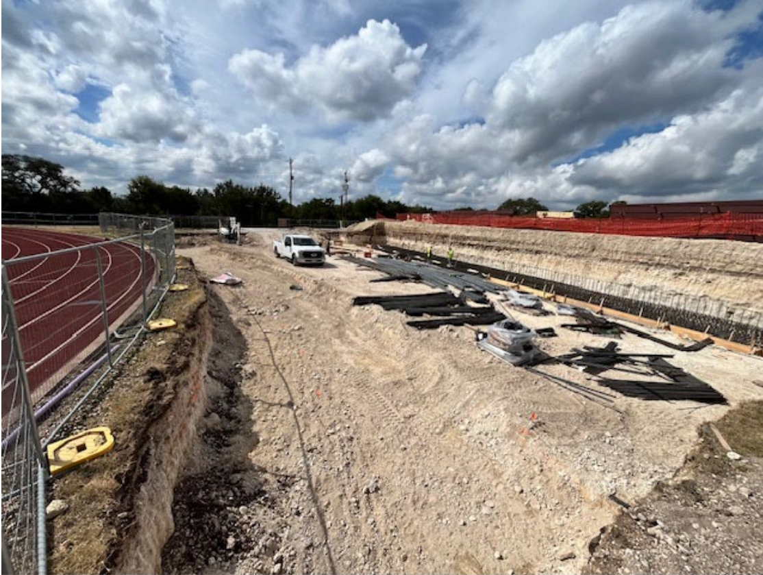
Photo: Underground Detention Pond
