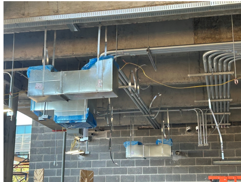
Overhead mechanical, electrical and plumbing 1 st floor
