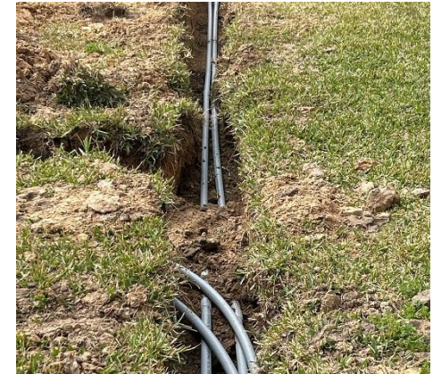
New site lighting power circuits installed.
