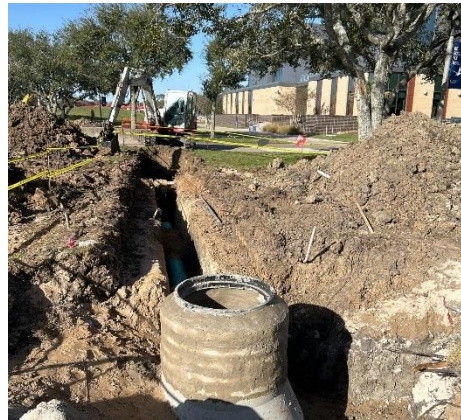
Sanitary sewer line mid campus.
