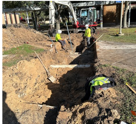
Sanitary sewer line mid campus.
