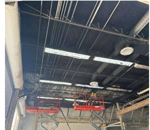
IE Building High Bay K-13 Insulation
