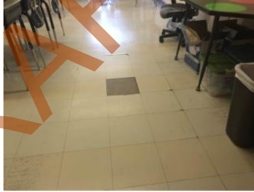
Missing and chipped VCT
