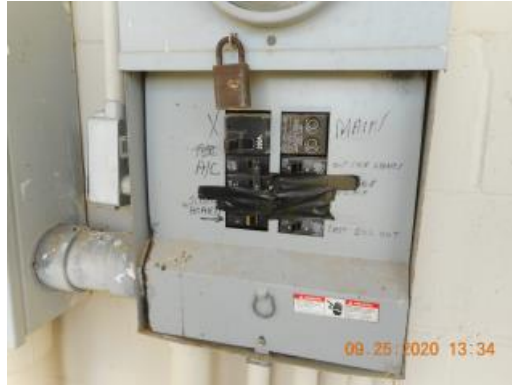
Panelboard with tape covering breaker switches
