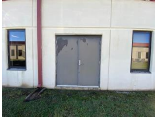
Worn exterior doors
