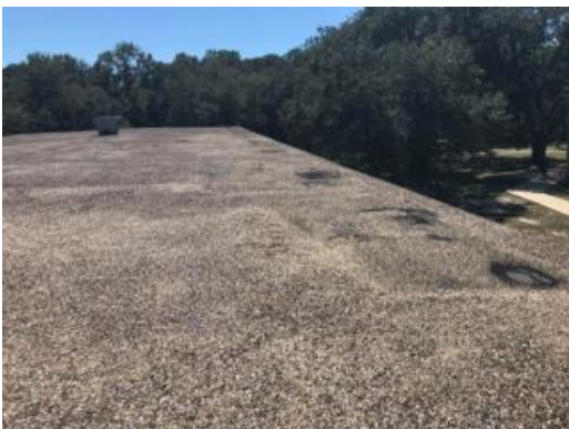
Built up roofing with evidence of leaks
