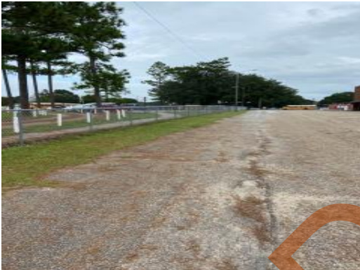
Asphalt to be replaced north of Bldg A
