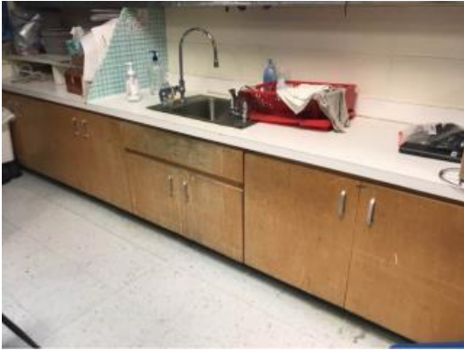
Worn classroom cabinetry
