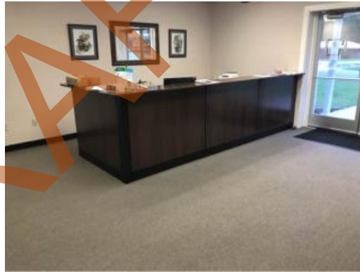
Lobby counter height not ADA compliant
