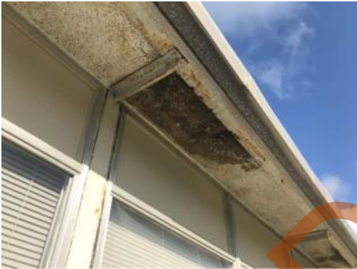
Building A soffit damage
