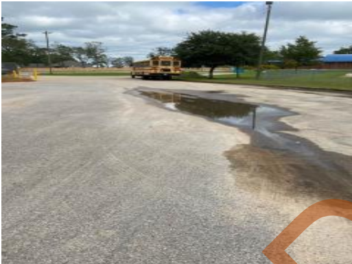
Ponding in east parking lot
