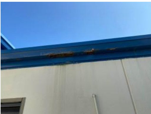
Rusted out gutters
