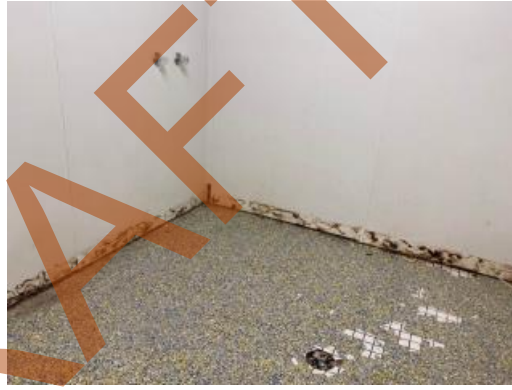
Damaged wall in group shower area
