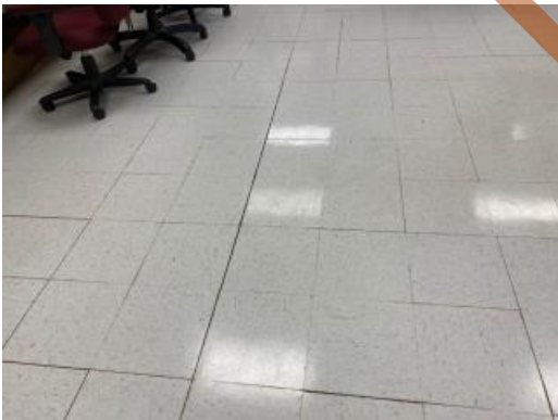
VCT separating at seams
