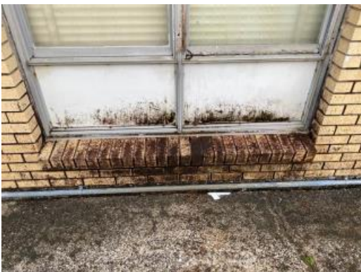
Dirty window sills
