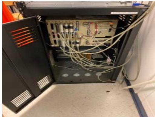
Obsolete PA system
