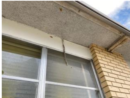
Failing caulk joints
