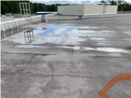
Ponding on roof
