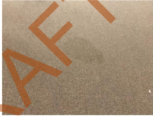
Water damaged carpet
