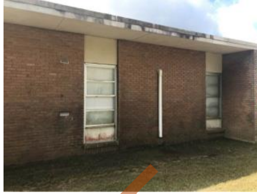
Building A old worn windows
