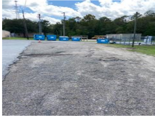
Failed asphalt west of cafeteria
