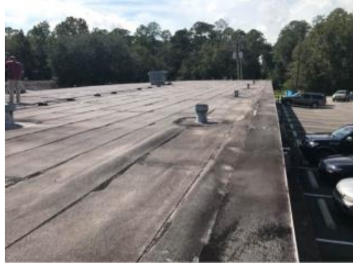
Delaminating mod bit roof
