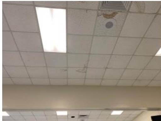
Water damaged ceiling tiles
