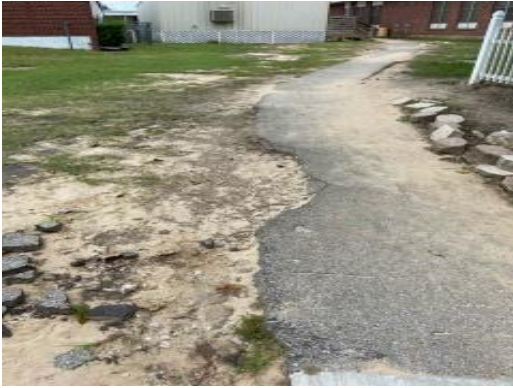
Failed asphalt walkway between Bldg F and H
