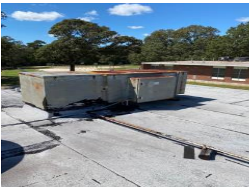
Abandoned make up air unit
