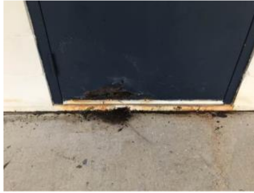
Rusted exterior door
