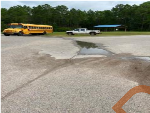
Driveway pavement failure
