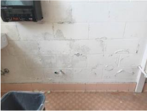
Peeling restroom wall paint
