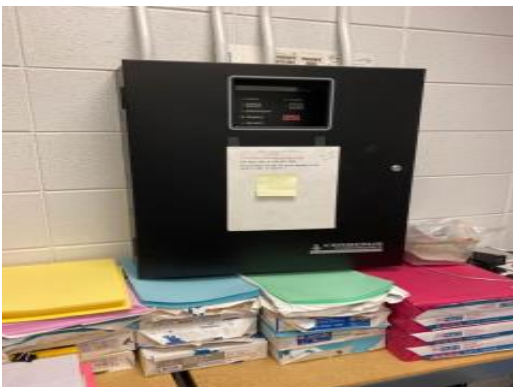
Obsolete fire alarm system
