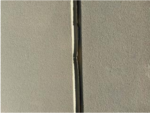
Concrete panel joint needs recaulking
