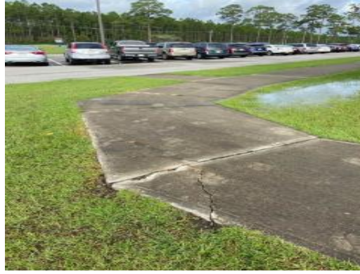
Damaged south sidewalk
