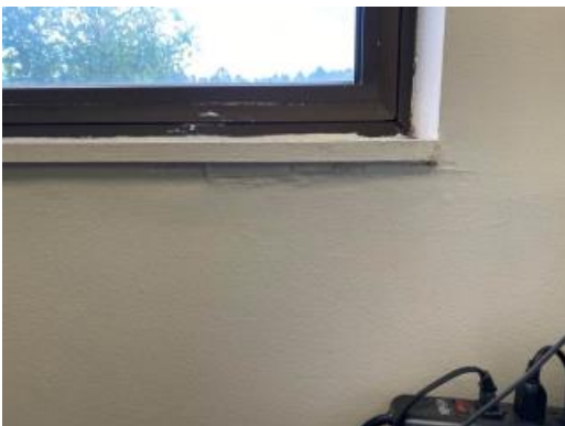
Water damage at leaking window
