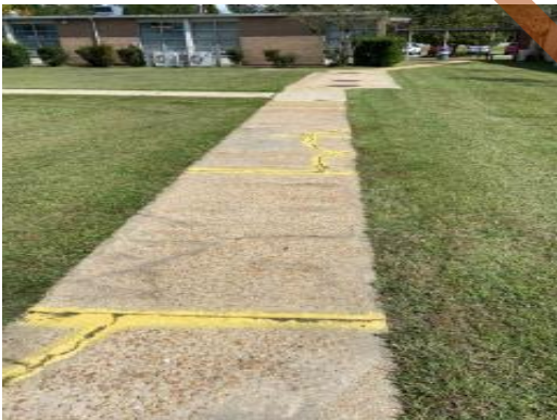
Cracked sidewalk in north courtyard
