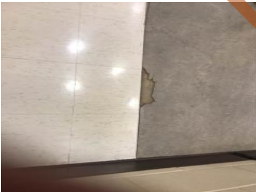
Worn hallway floor
