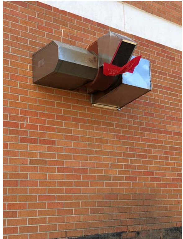
Vent hood on west wall of north building must be moved
