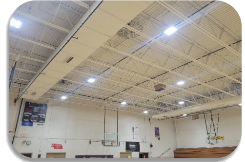
High School Gold Gym Ductwork and Sprinkler Piping – Remove in their Entirety
