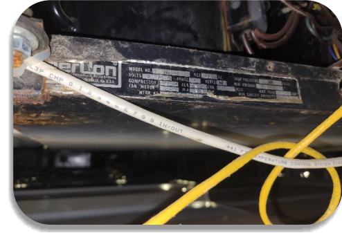
Hayward Water Source Heat Pump – Circa 1977
