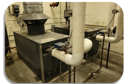
High School Camus Boilers, circa 2010
