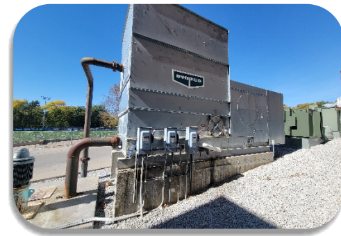
High School Cooling Tower, circa 2010
