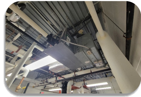
Northside Mechanical Room Water Source Heat Pump - 2009
