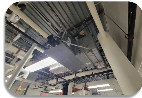
Northside Mechanical Room Water Source Heat Pump - 2009
