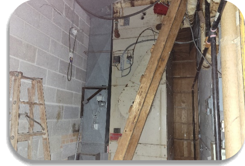
High School Old Gym AHU, circa 1967 (Offline)
