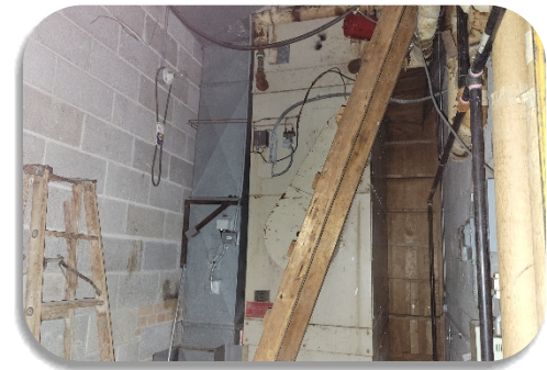
High School Old Gym AHU, circa 1967 (Offline)
