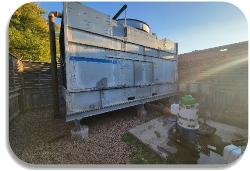
Middle School Cooling Tower - circa 2004
