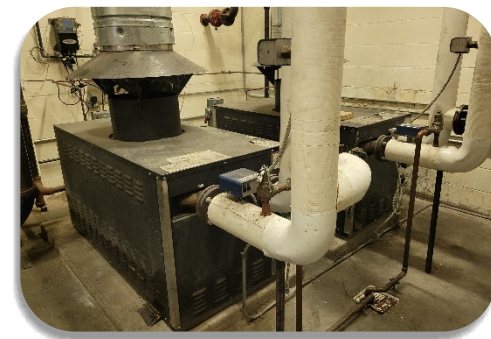
High School Copper Tube Boilers, circa 2010
