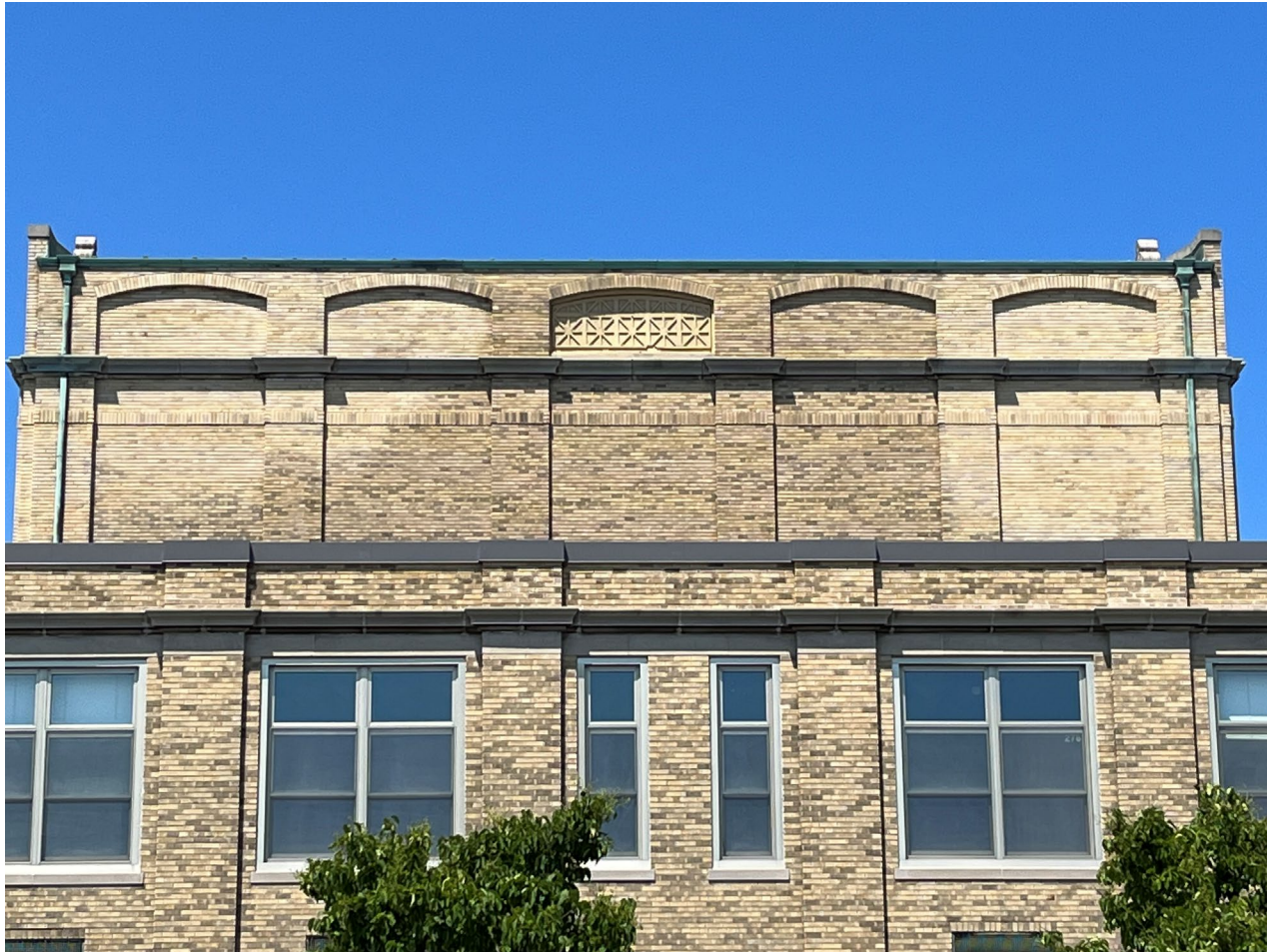
Difference in existing versus cleaned (upper corners cleaned)
