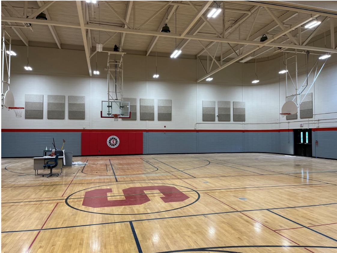
Gym lighting, acoustical tile and painting complete. Floor to be re-sealed August 28 th
