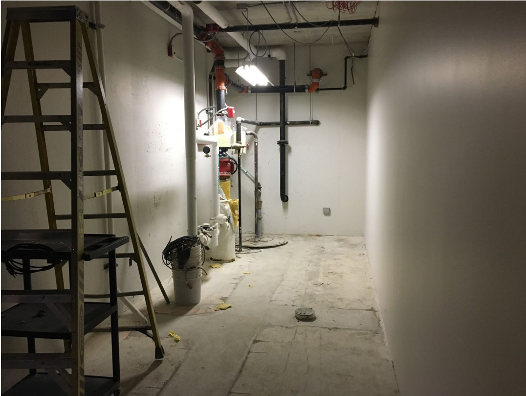
Newly created fire-pump room
