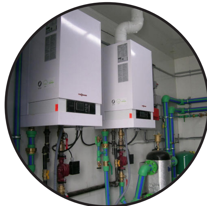
High-Efficiency Mechanical Systems Reduce Energy Loads
