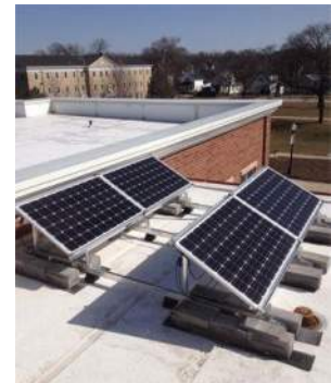
Photovoltaic panels at Elgin Academy
