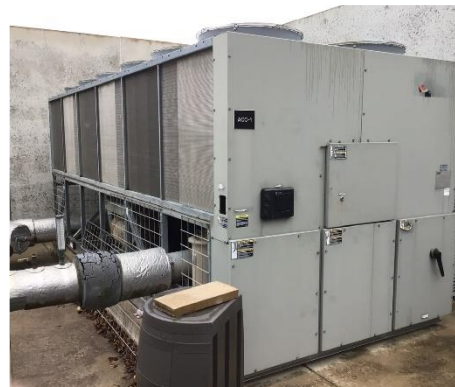
Air Cooled Chiller
