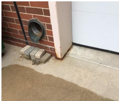
Rusted frames on exterior
