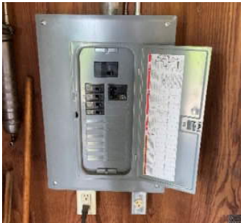
Existing Electrical Panel
