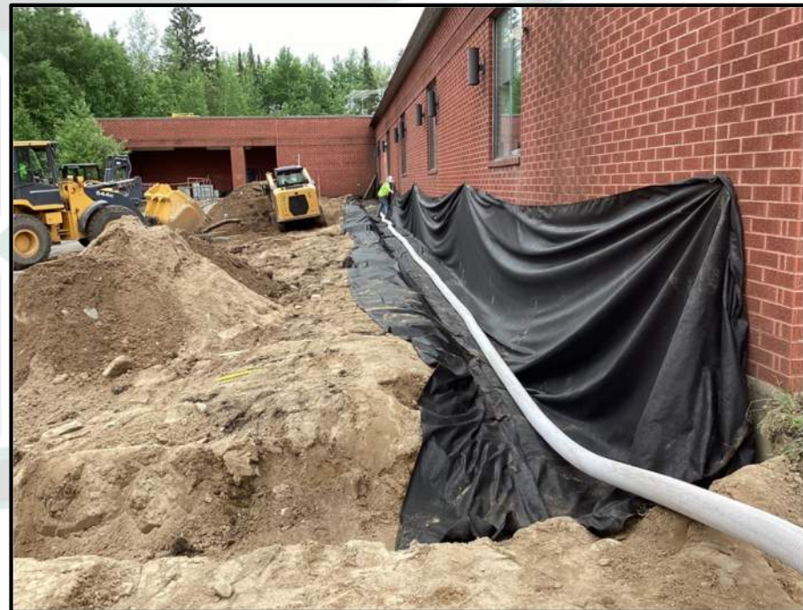
Installing drain tile and washed rock to direct water away from the building.
