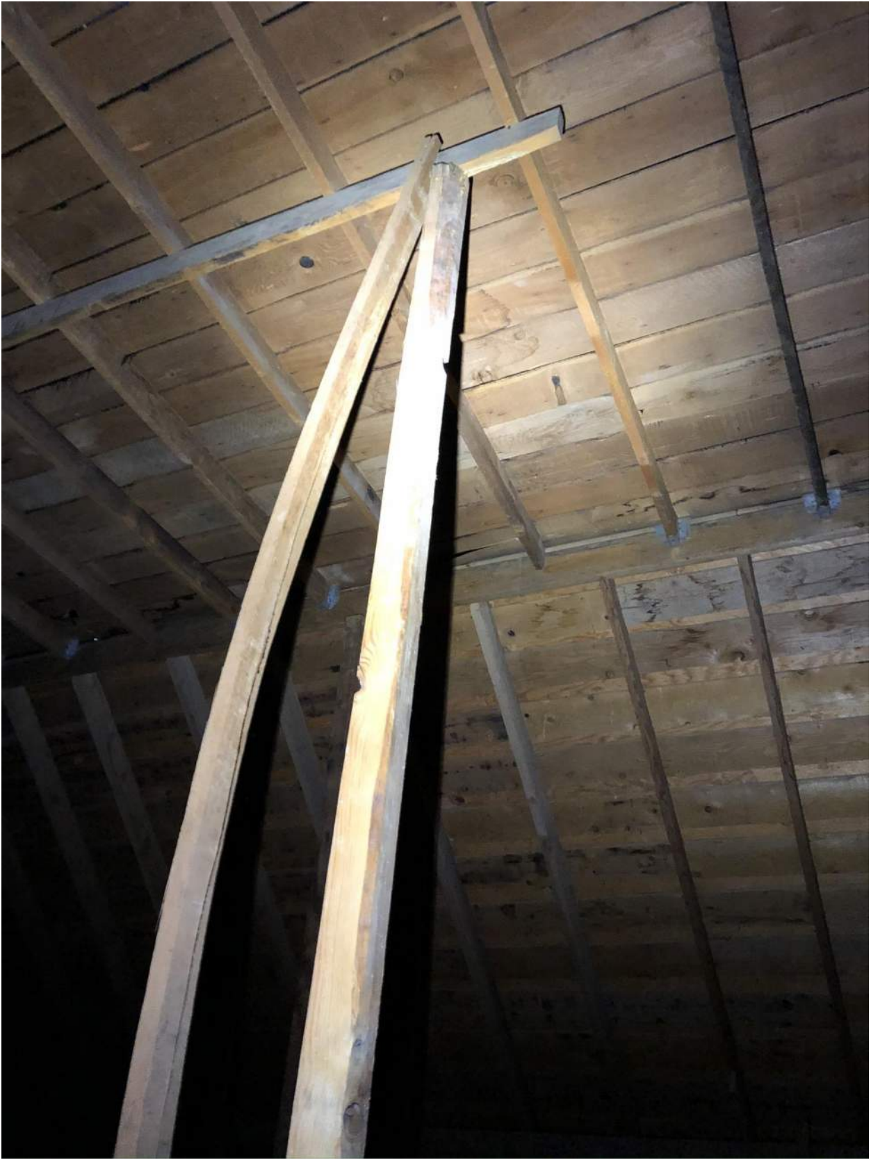
Photo 5 - Existing roof framing over classroom area. Note buckled and bowed bracing member.
