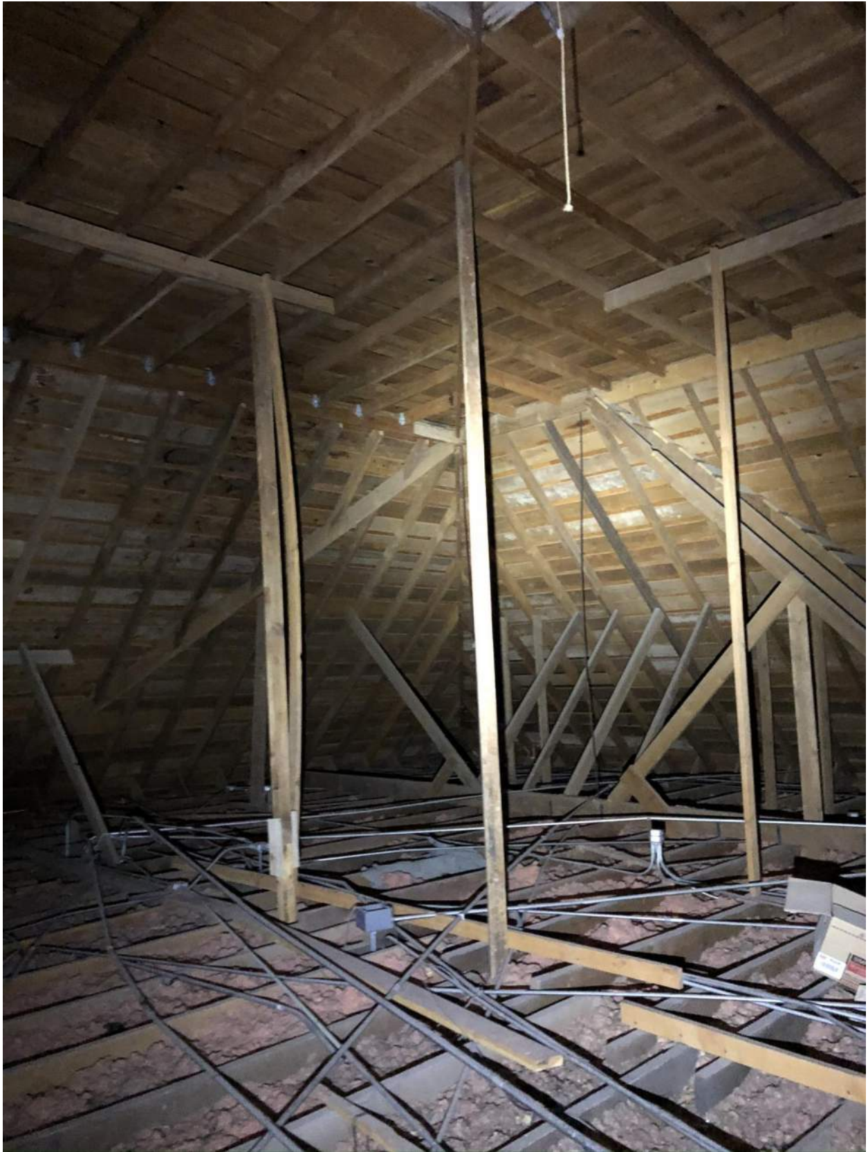
Photo 4 – Existing roof framing over classroom area. Note erratic, inadequate support and bracing.
