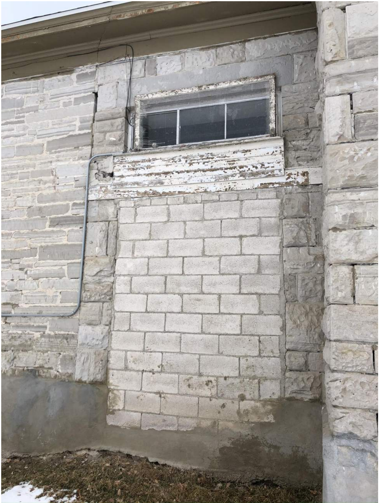
Photo 15 – View of infilled opening in south exterior wall. Note the wood header below the window, which is deteriorating.
