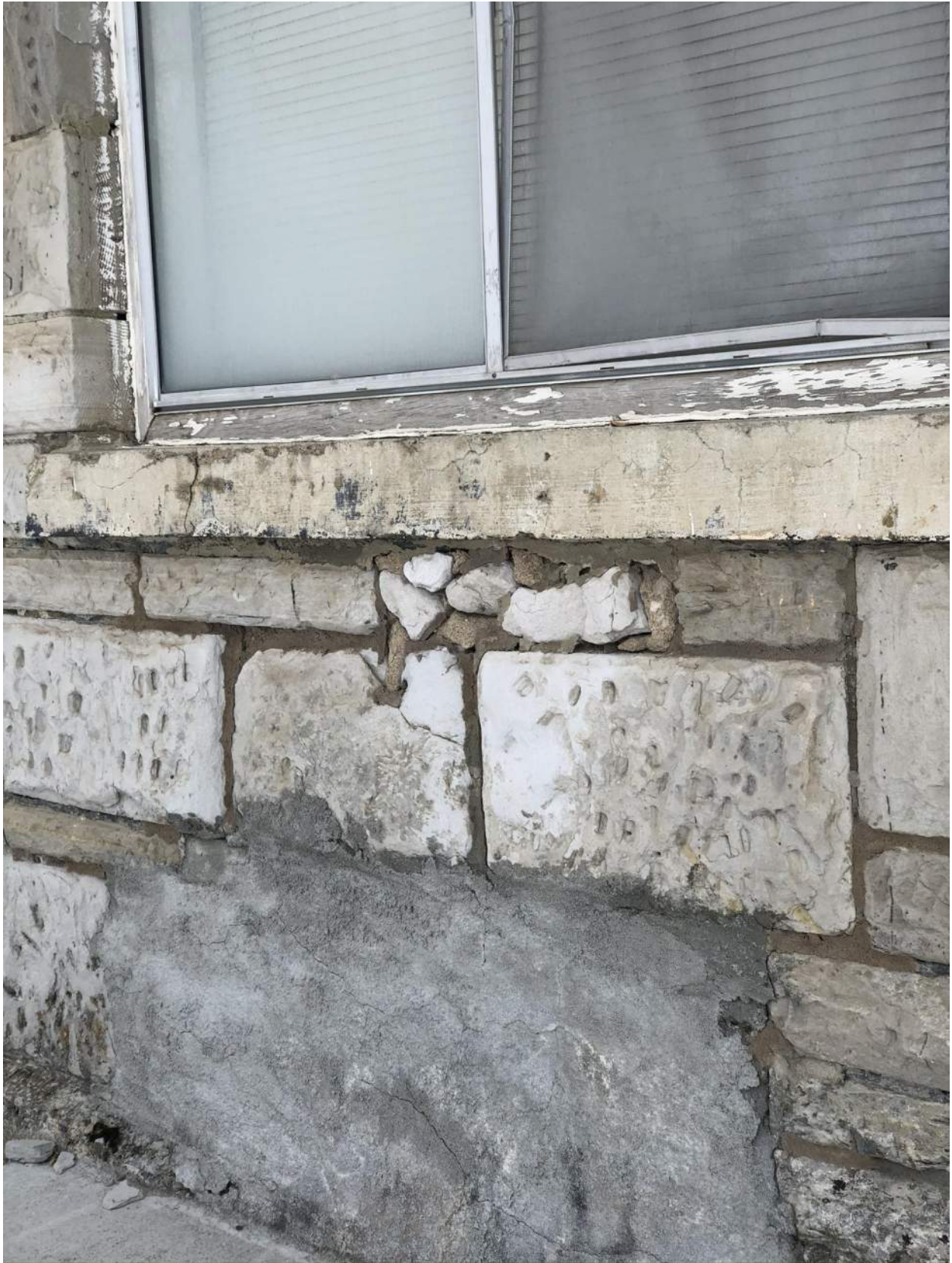
Photo 16 – View of stone and deteriorating mortar along the north exterior wall.
