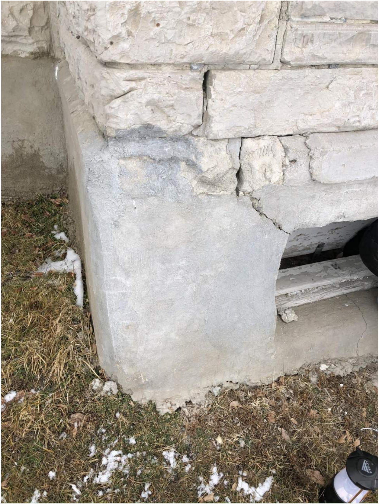
Photo 13 – View of foundation along the south wall. Settlement and cracking are present.
