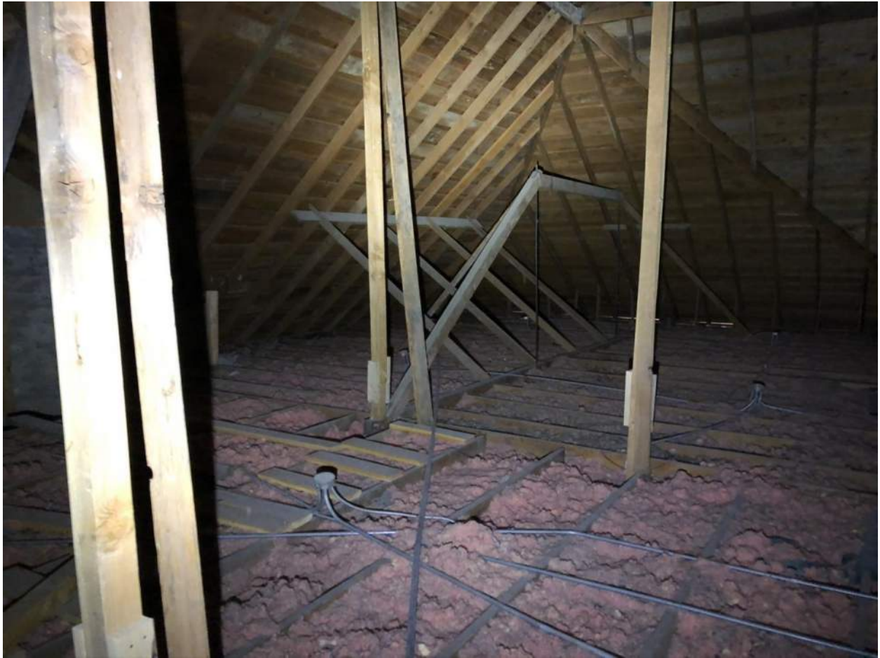
Photo 12 – View of wood and steel rod attic truss for ceiling joist support. This truss is clearly inadequate for its intended use.
