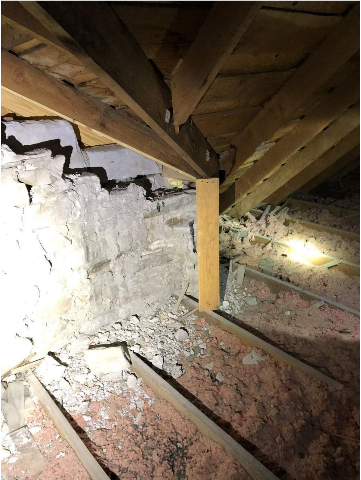
Photo 8 - View of inside face of gabled end wall above east entry. This is the condition at the base of the roof valley. Inadequate brace and support.
