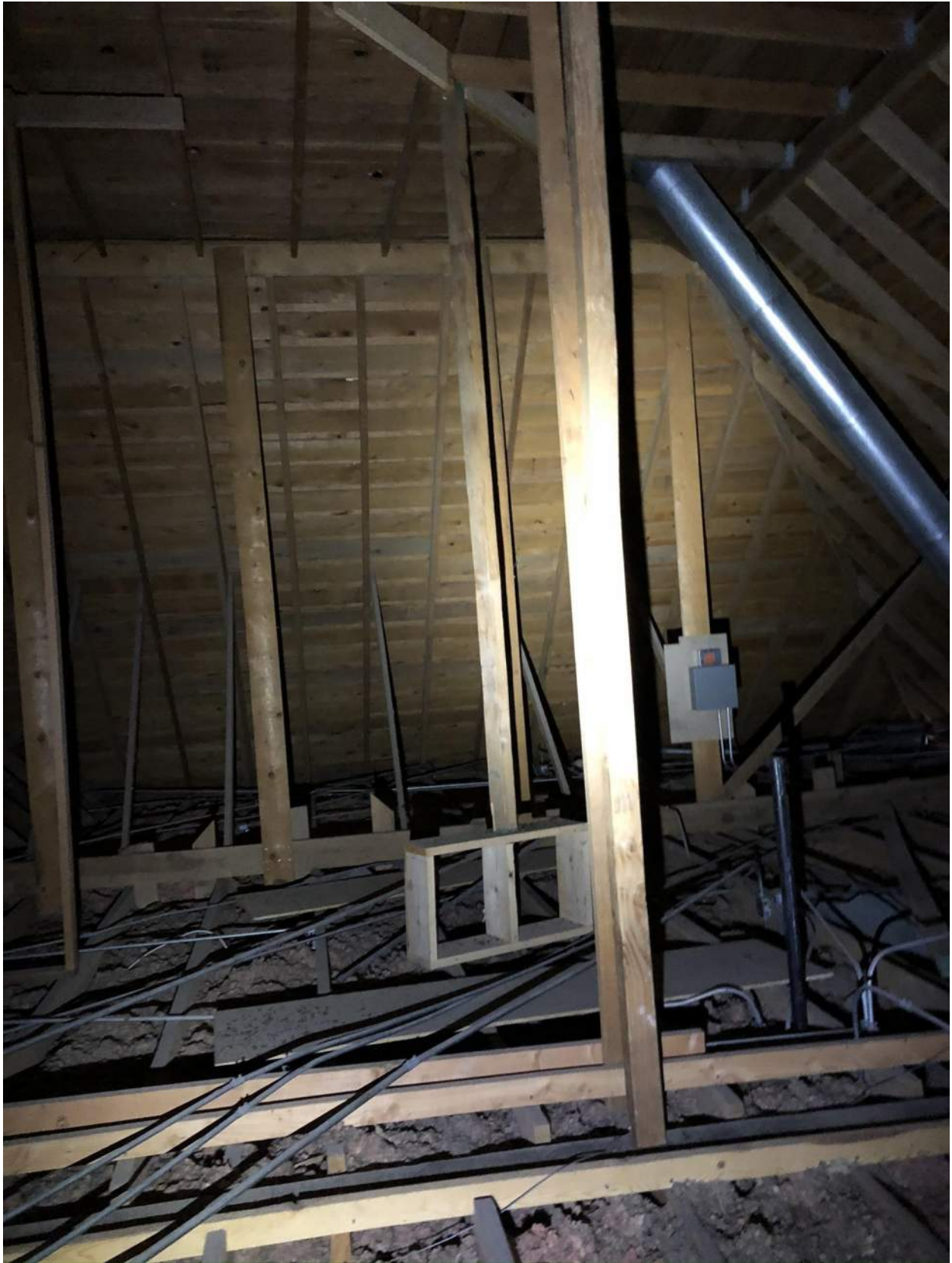
Photo 6 - Existing roof framing over classroom area. Note erratic, inadequate support and bracing.
