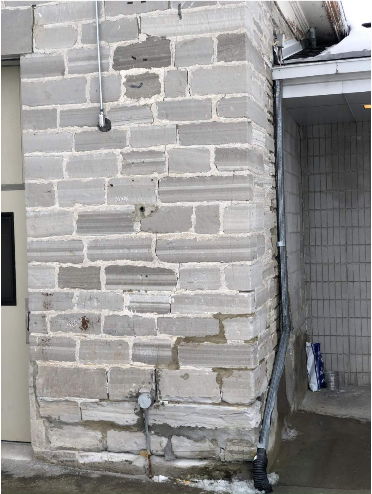
Photo 18 – View of the northwest corner of the kitchen area, near the breezeway. Note mortar deterioration and cracking.
