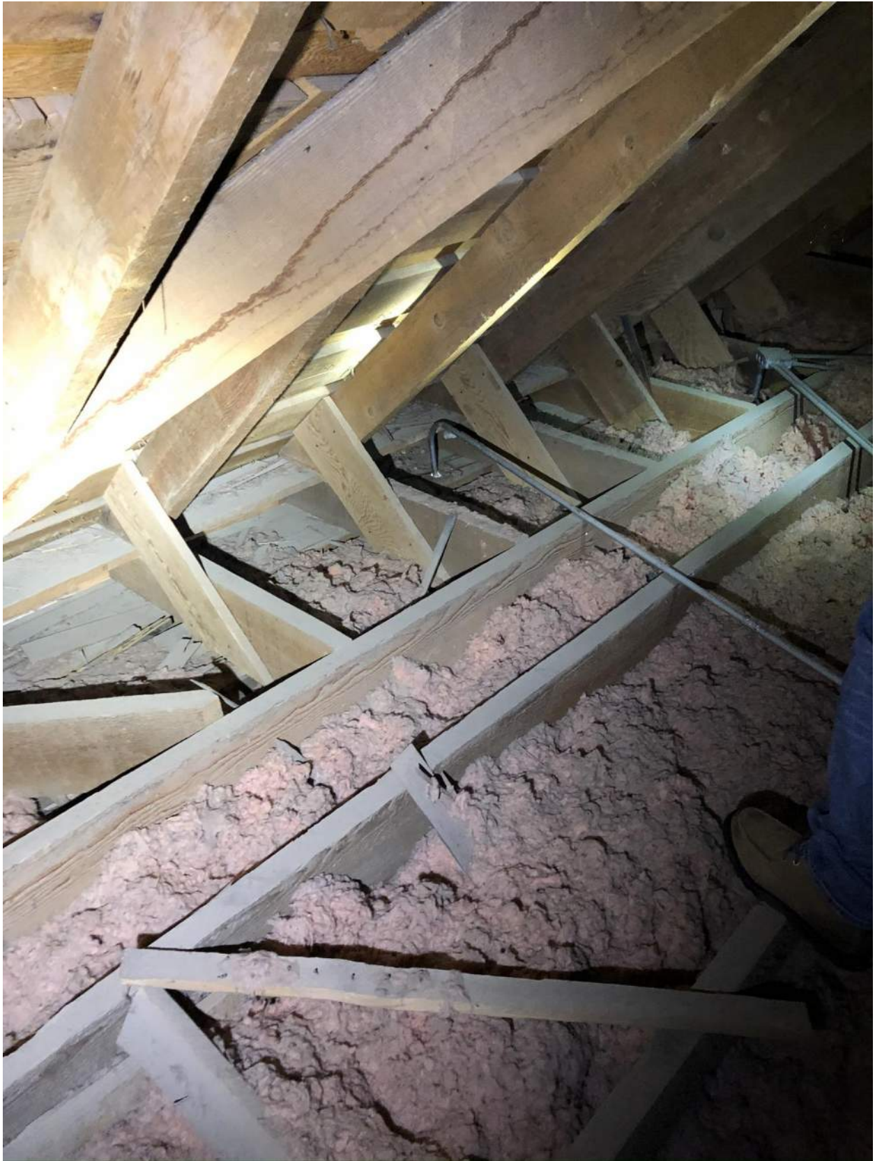
Photo 9 – View of roof to wall connection along north and south exterior walls. No in-plane shear connection or out-of-plane anchorage to the stone wall below.
