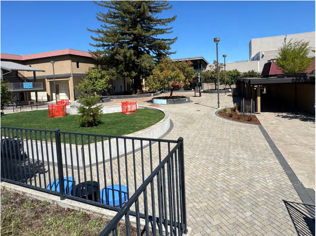
AHS Quad Renovation with post Seismic Retrofit Science Building in the backdrop!
