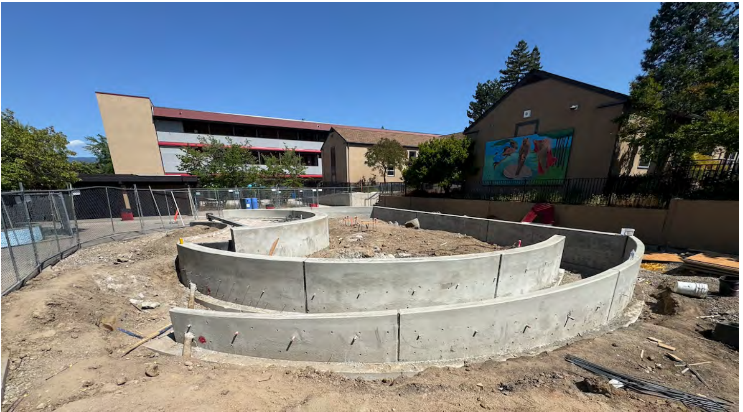
Ashland High School site wall concrete at the new raised lawn area in the quad!
