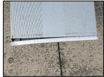
Loose/damaged end cap.
