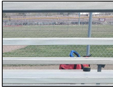
Gaps between planks exceed 4" standard.
