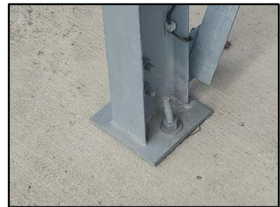
Concrete ground anchor.
