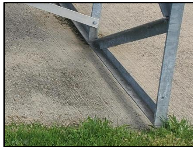
Missing ground sill.
