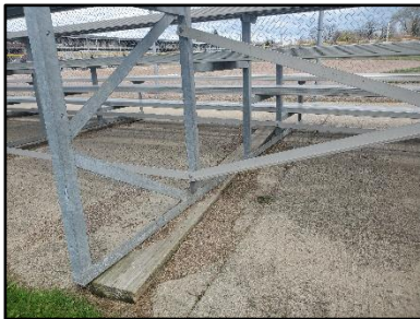
Misaligned/bent frame member.
