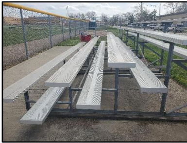
Missing side/rear guardrail fencing.
