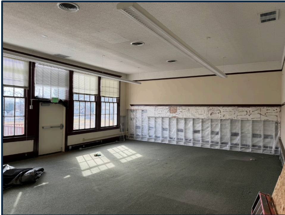
Subject former classroom space (with deferred maintenance)
