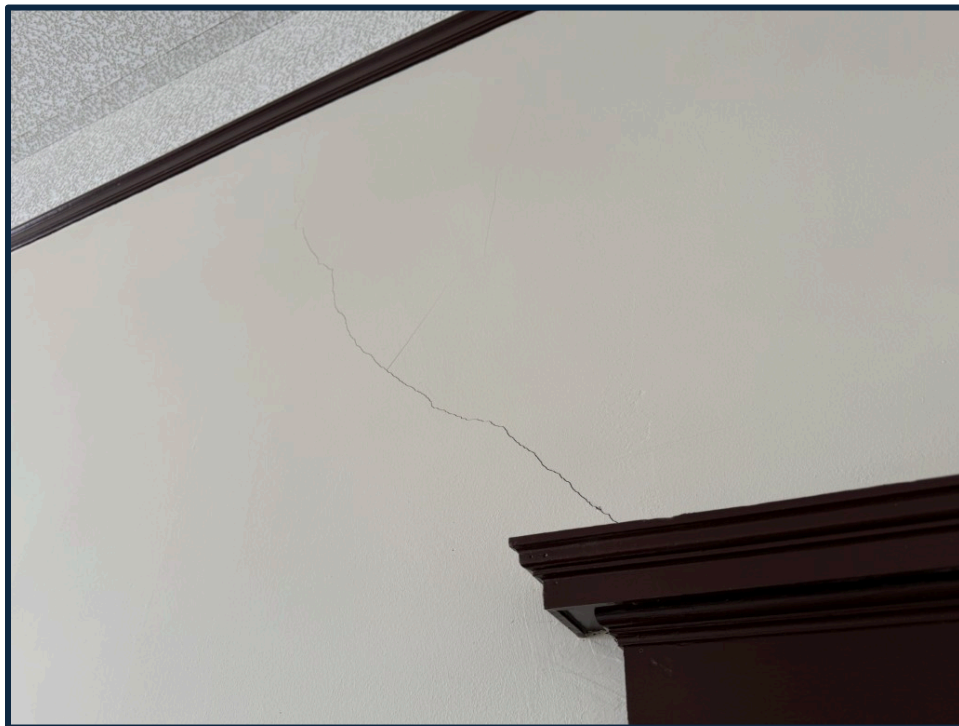
Subject deferred maintenance
