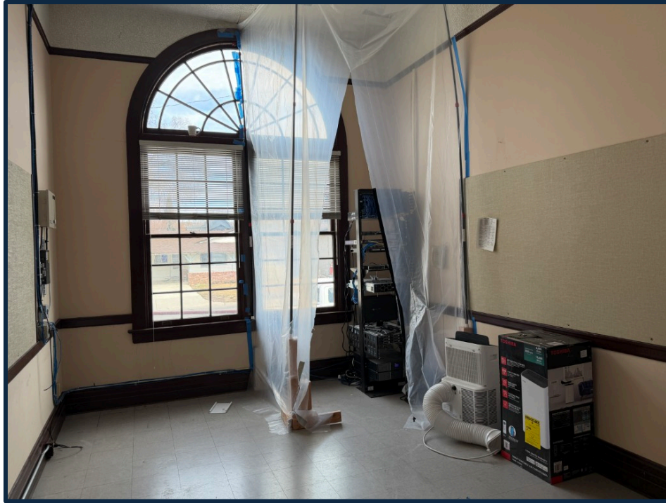
Subject deferred maintenance
