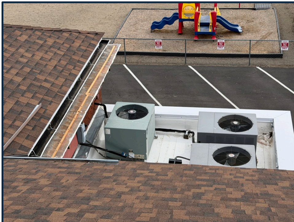
Subject condensing units
