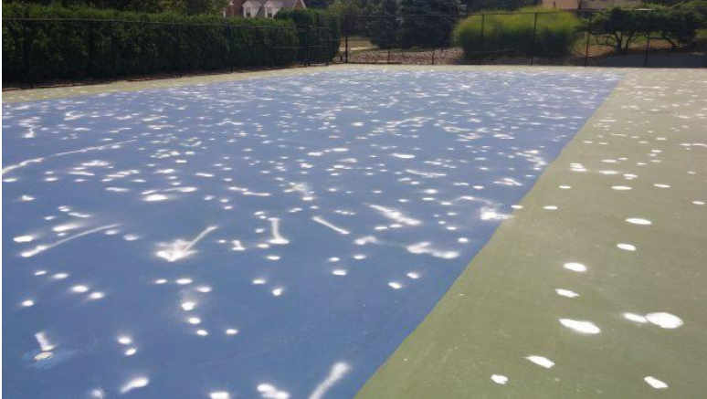
Rust Spots (Acrylic Patch After Removal of Rust Spots)
