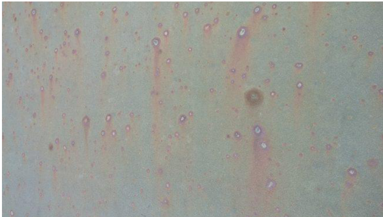
IRON PYRITE RUST SPOTS AND STAINING
