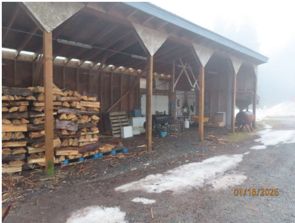
Cord wood boiler and wood storage structure
