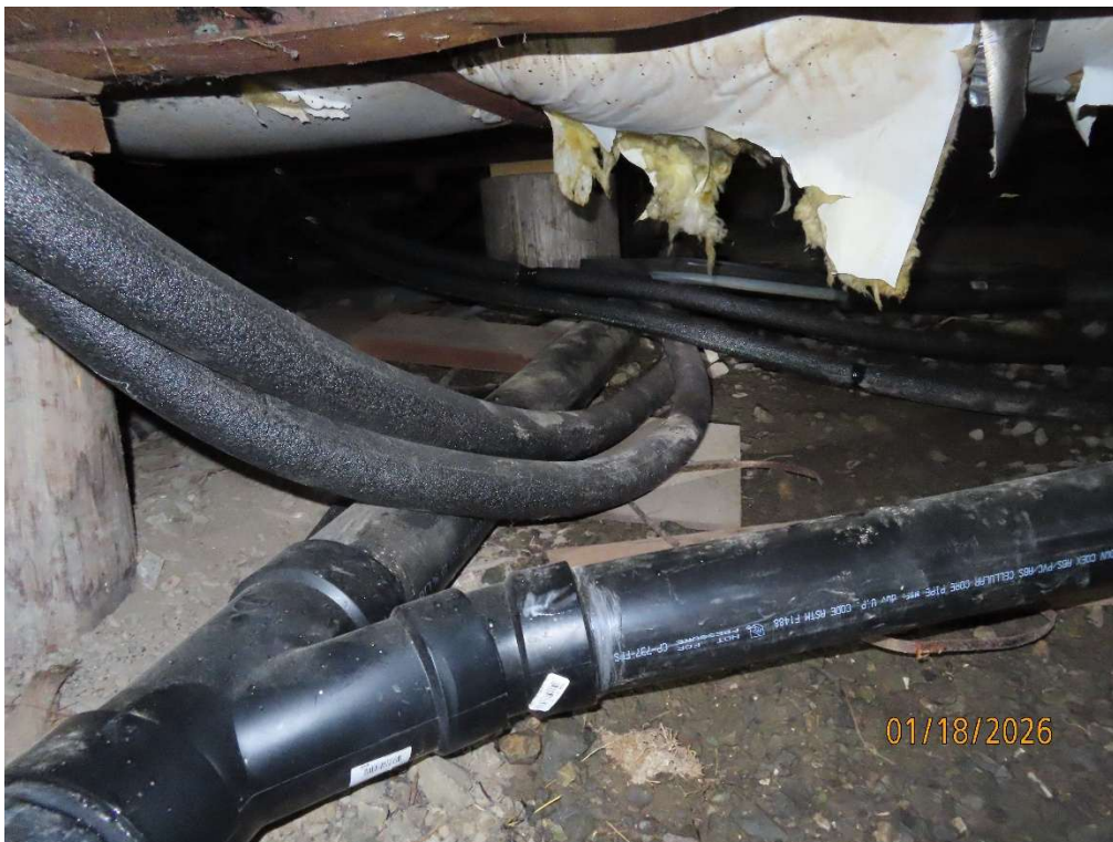
Insulated PEX tubing connecting hydronic wall heaters to the cord wood boiler
