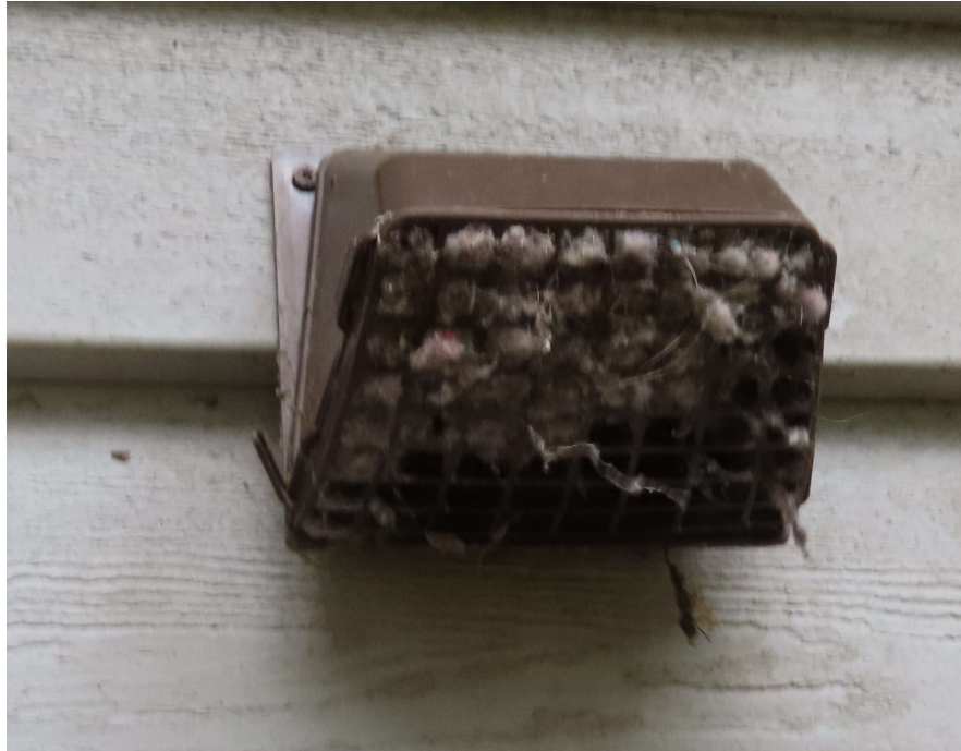
Clogged dryer vent
