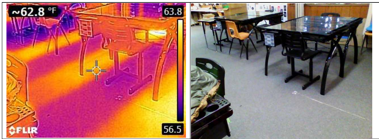
4. Substantial heat loss from uninsulated forced air heat ducting in the crawl space
