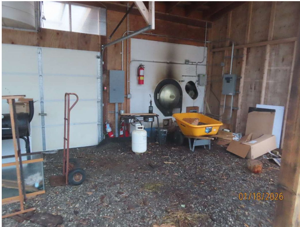
Garn cord wood boiler
