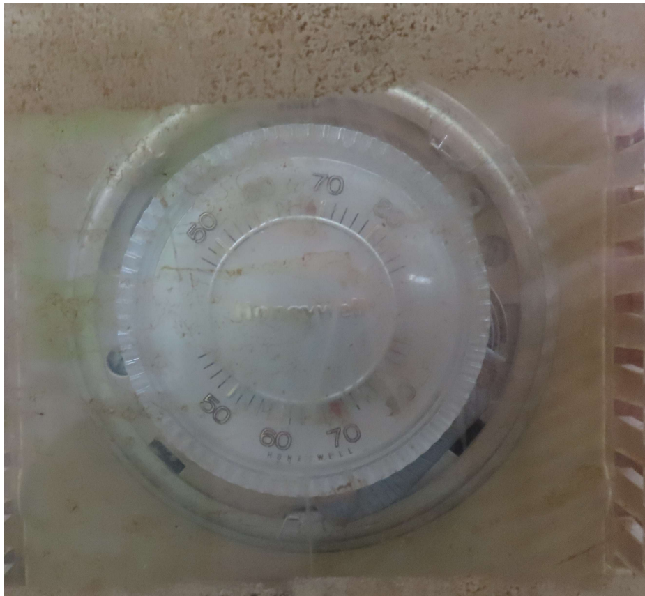
Elementary school thermostat in lockbox
