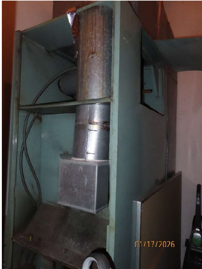
40+ year old furnace in elementary school
