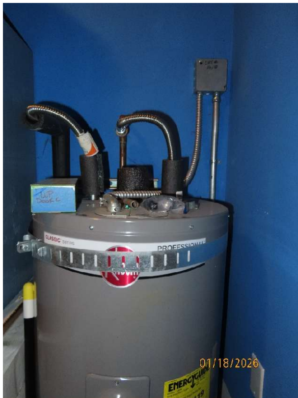
Hot water heater located in storage closet
