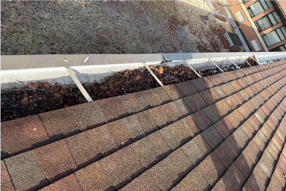
Typical leaves and ponding water in gutter.
