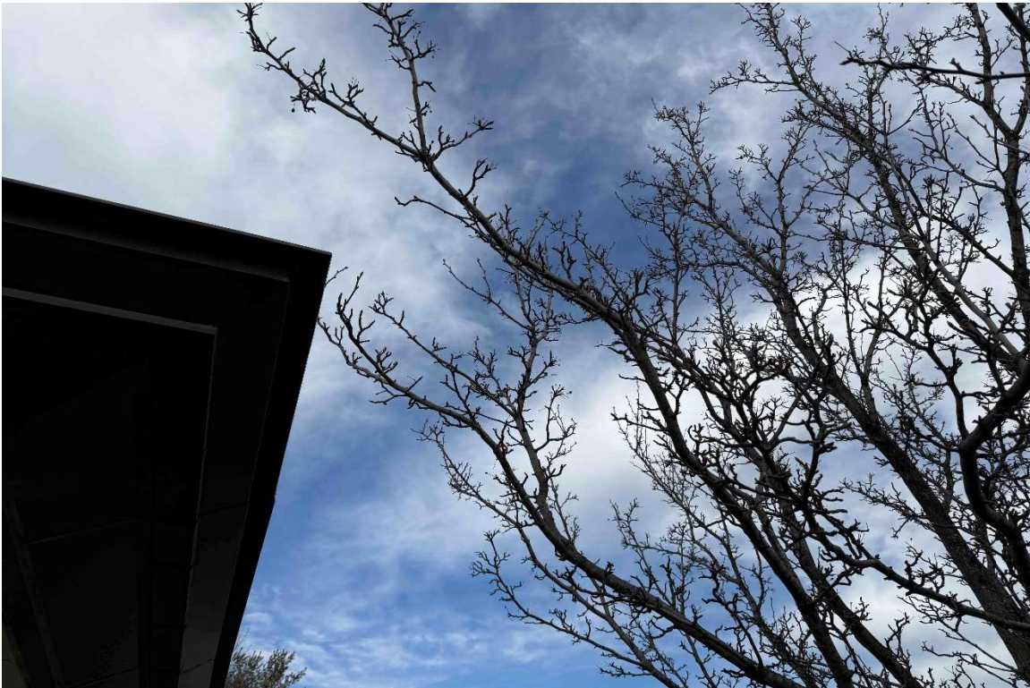
Rodent access point due to overgrown trees.
