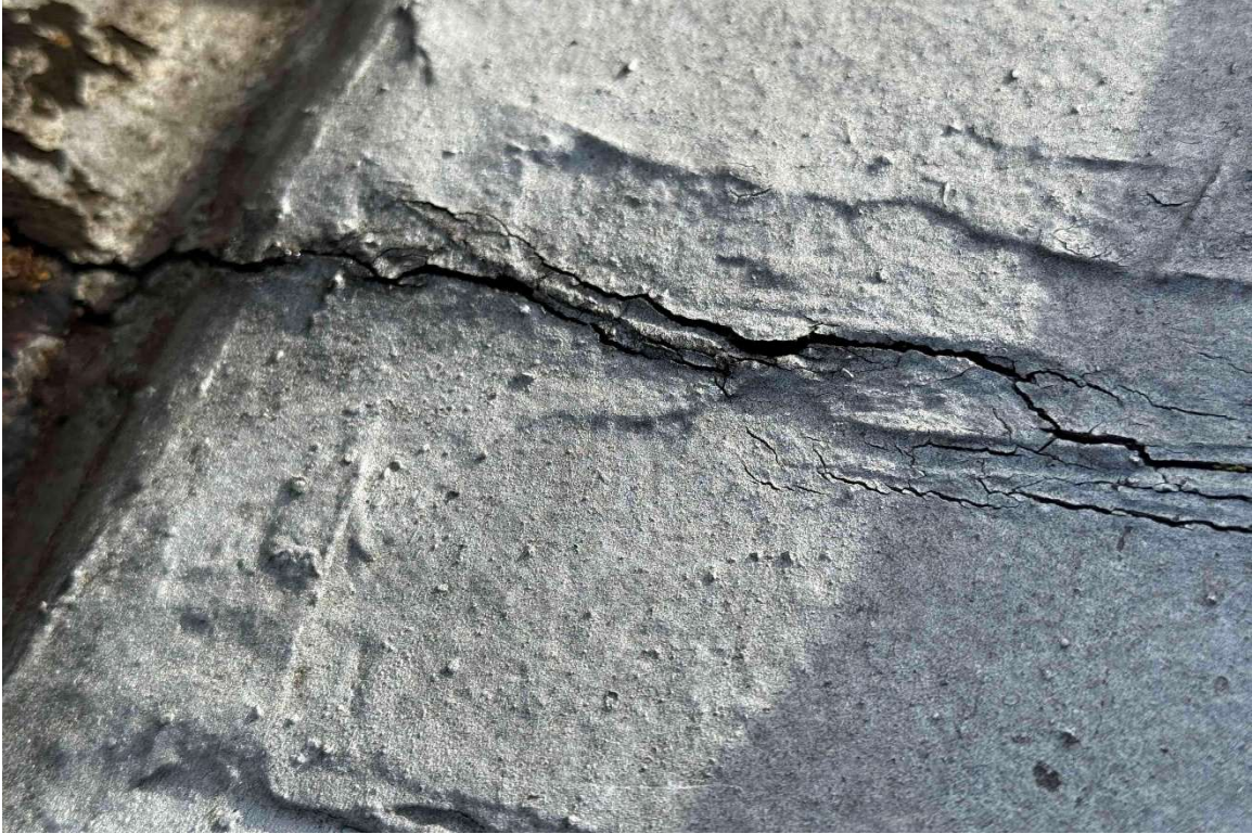
Splits located at existing gutter repairs.
