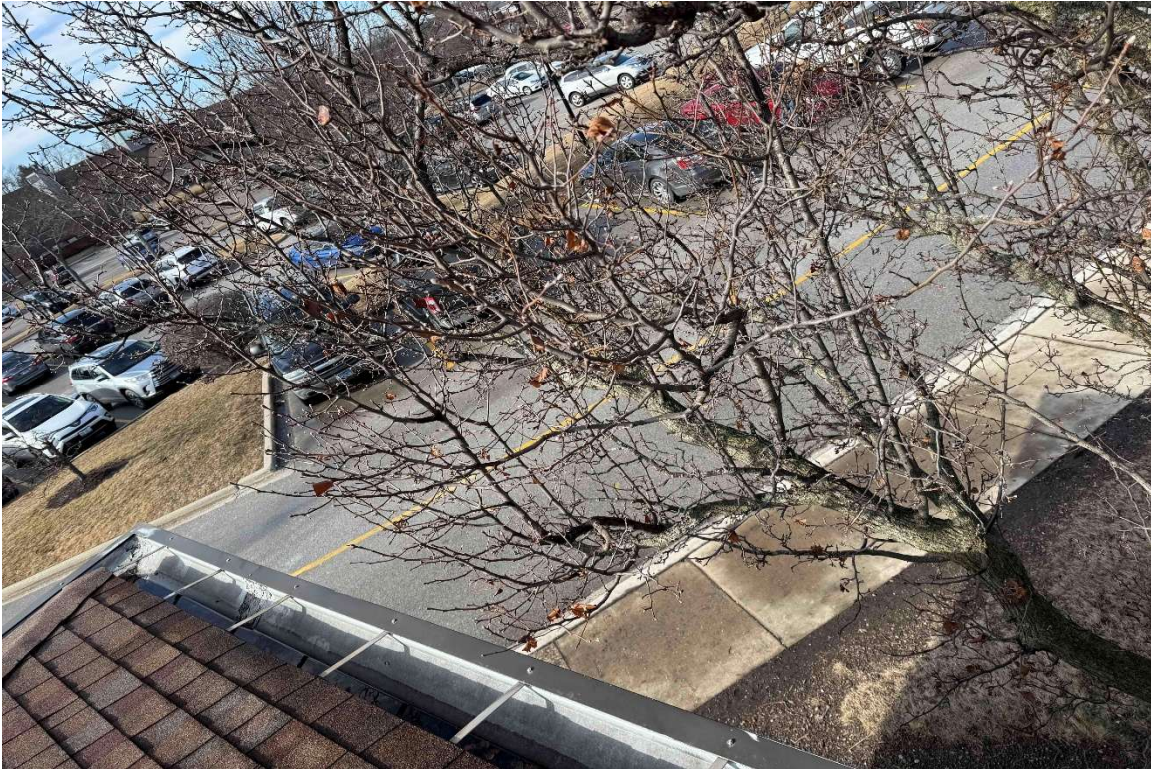
Rodent access point due to overgrown trees.
