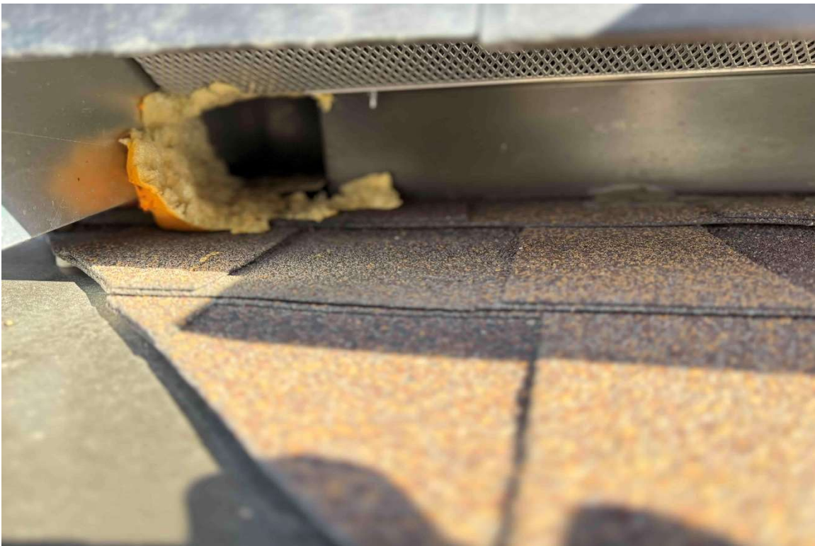
Rodent entry point at open roof vent.
