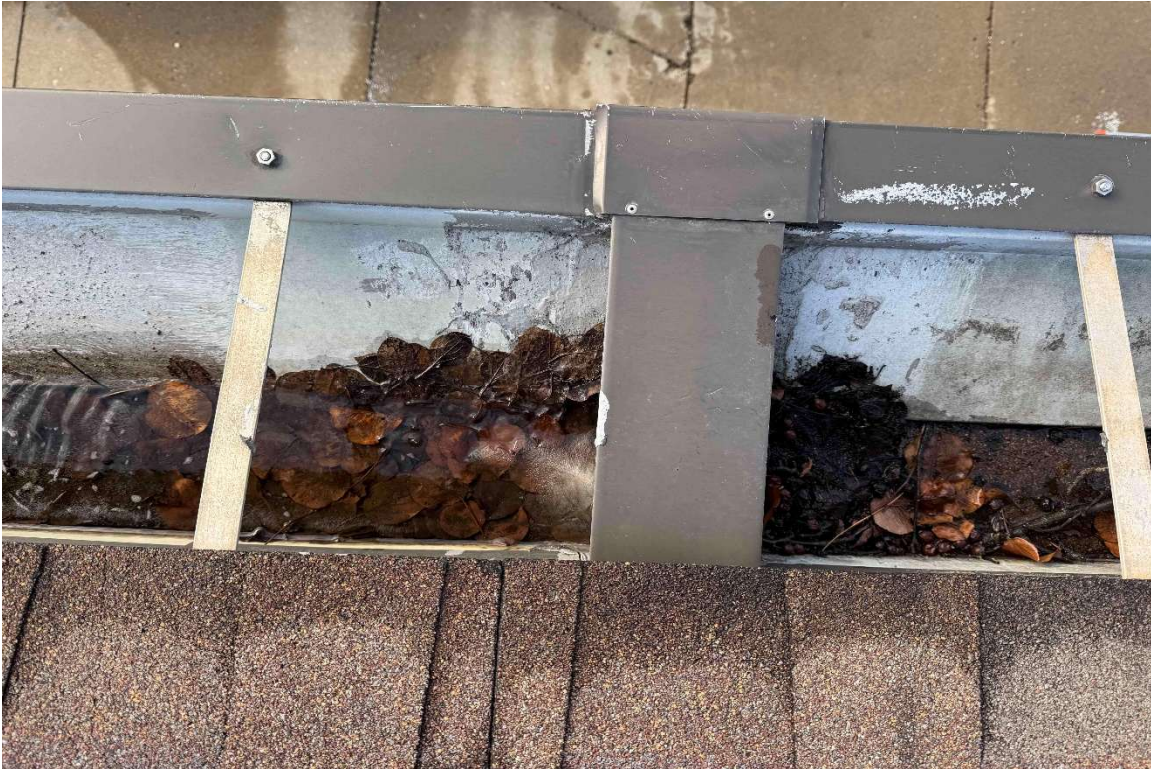
Typical leaves and ponding water in gutter.
