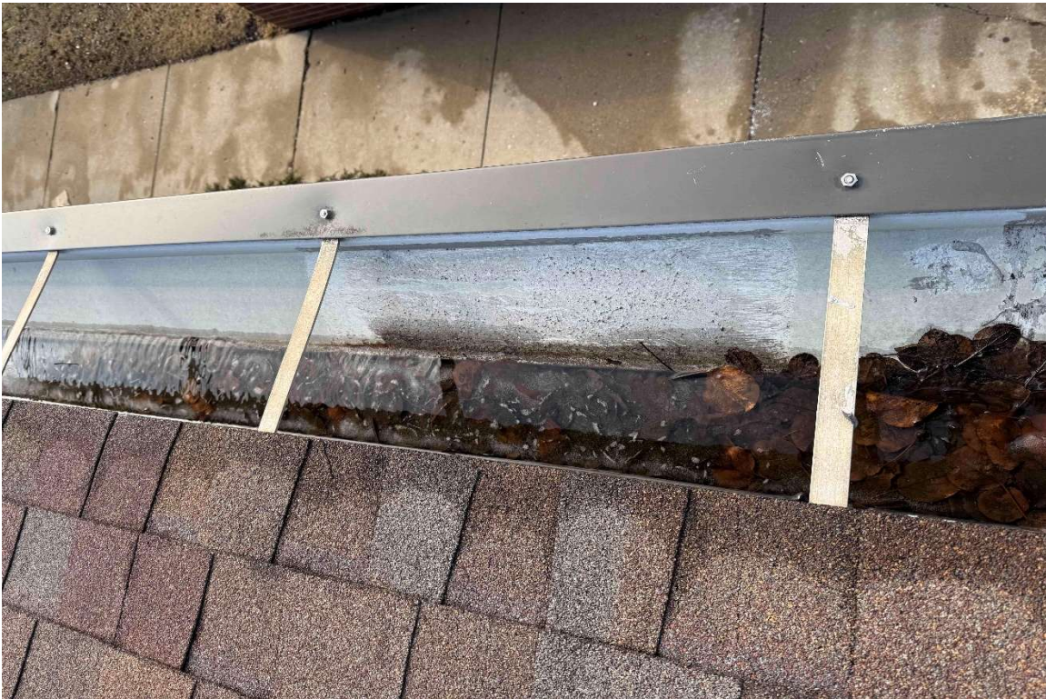
Typical leaves and ponding water in gutter.
