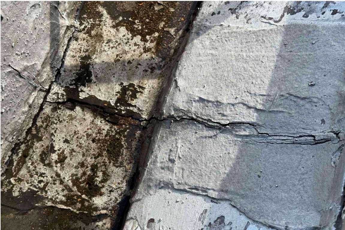
Splits located at existing gutter repairs.
