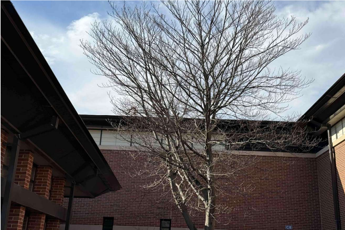
Rodent access point due to overgrown trees.
