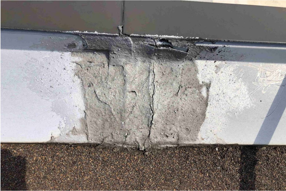
Splits located at existing gutter repairs.
