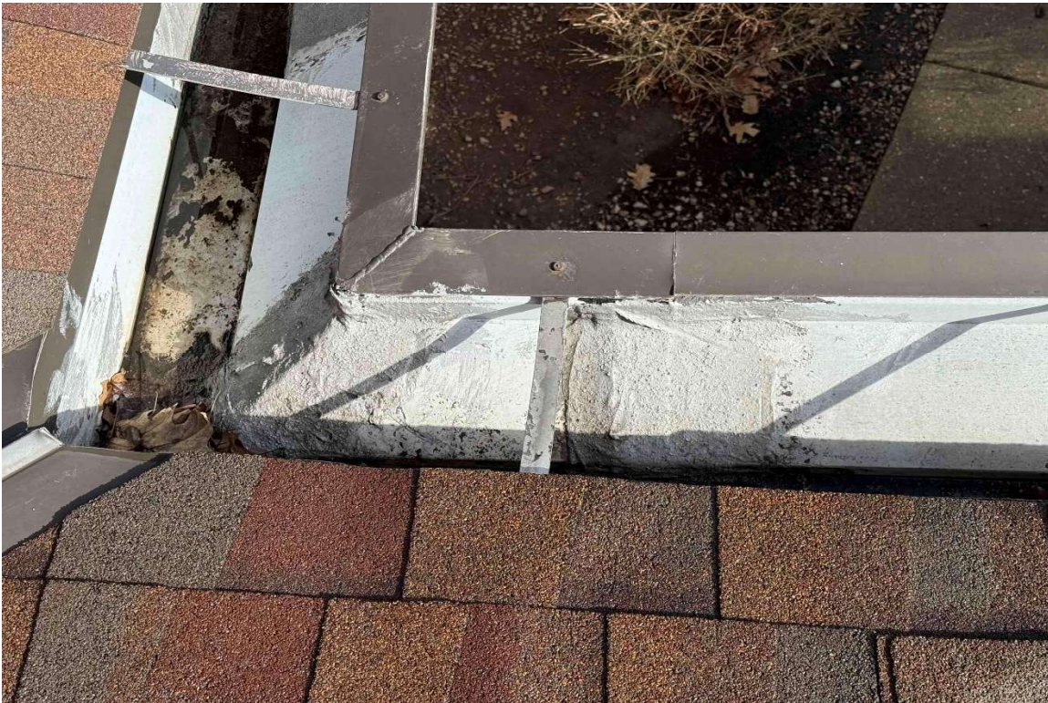
Splits located at existing gutter repairs.
