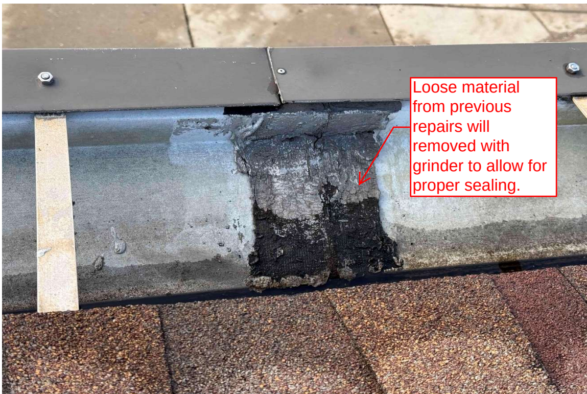
Splits located at existing gutter repairs.
