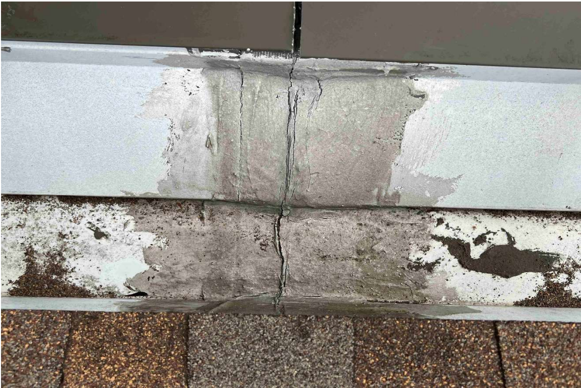
Splits located at existing gutter repairs.
