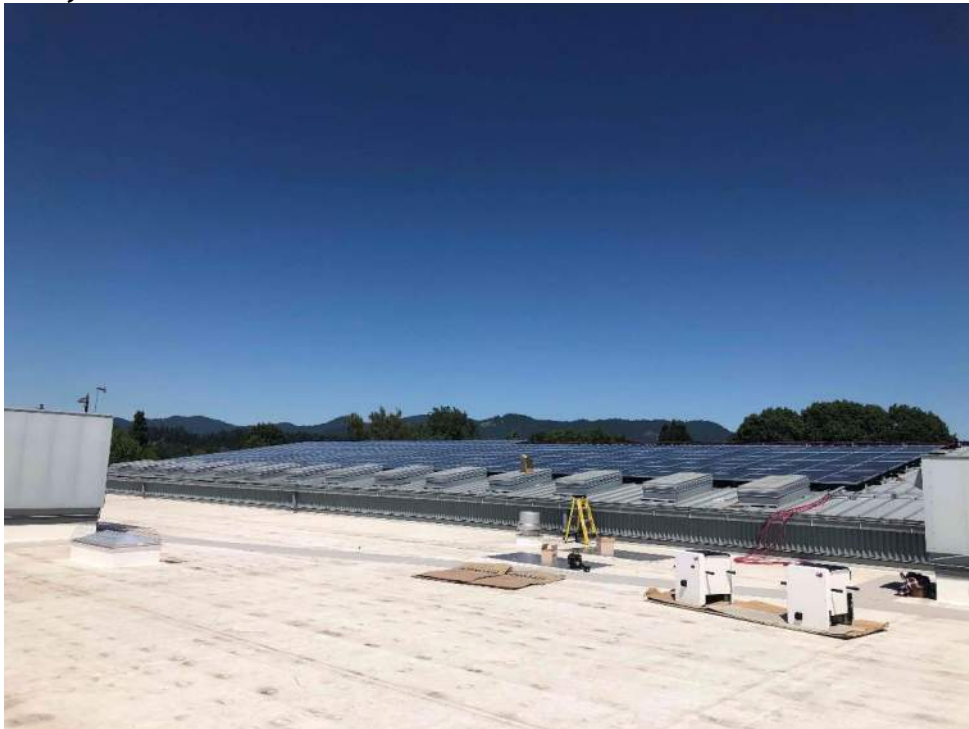
CHS – Largest solar array 95% complete over library
