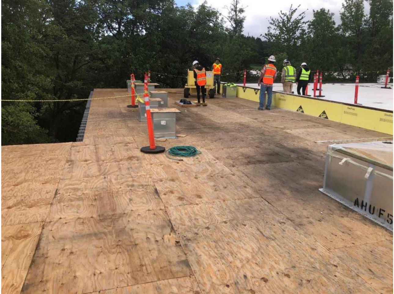
CVHS Building F – Roof deck ready and curbs are set and ready for finish roofing
