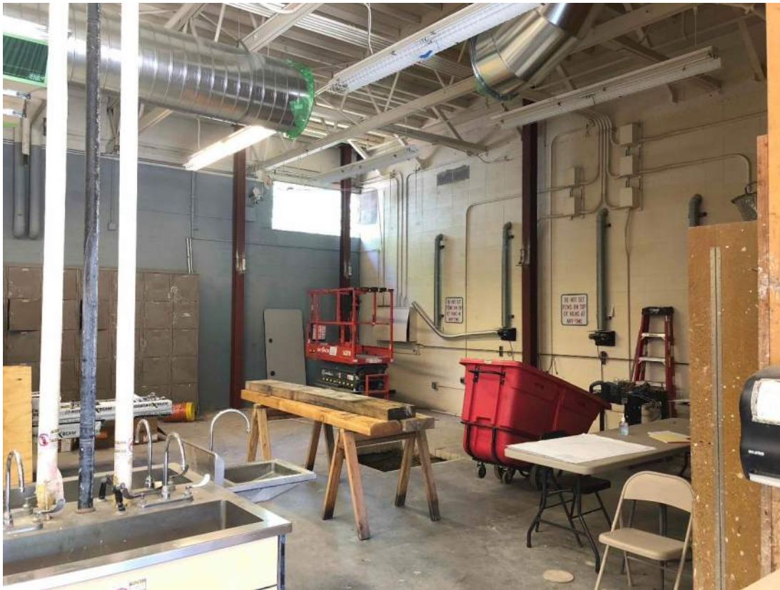
CHS - HVAC supports in ceramics
