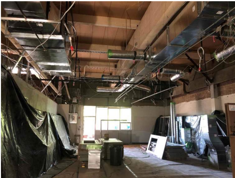
CVHS Building F – Jewelry HVAC
