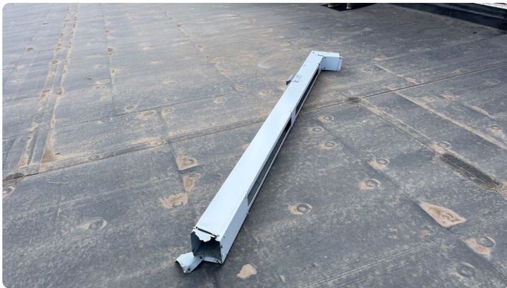
Photo showing downspout detached from Area 15 roof.
