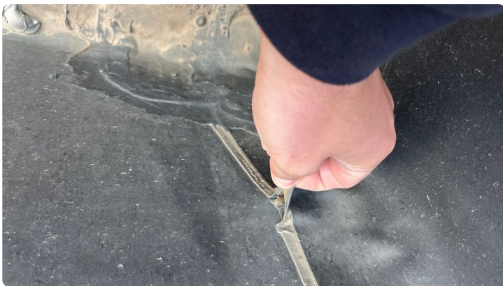
Photo showing an open wrinkle in the inside corner flashings causing a leak.
