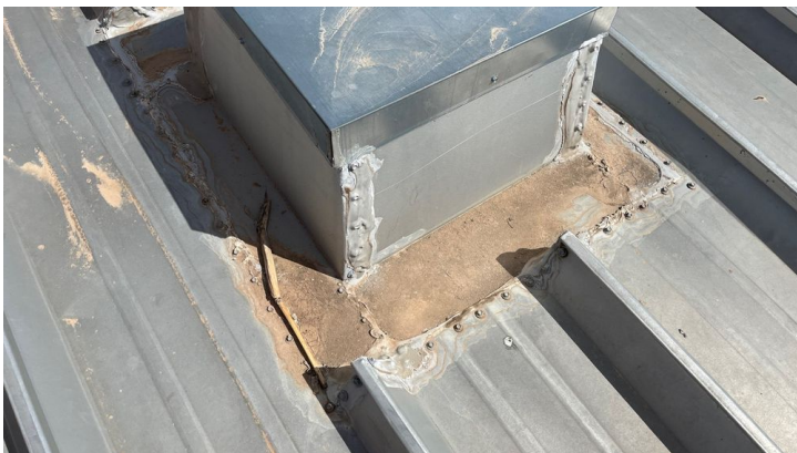
Photo showing sealant used throughout roof that is deteriorating around seams and flashings.
