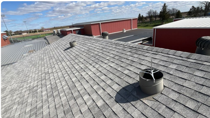
Photo showing two missing turbine caps.
