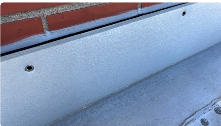
Photo showing missing chimney flashings fasteners.
