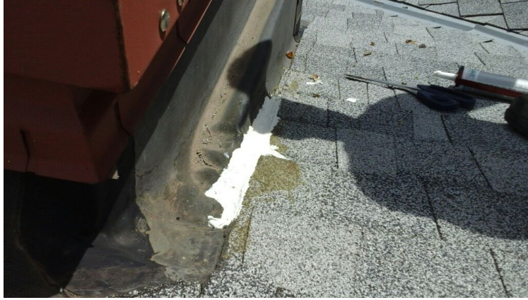
Photo showing temporary repair made to the hatch where silicone was pulled up.
