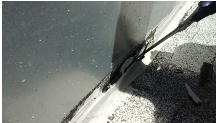
Photo showing failing flashings along curb. Caulking pulls right up which means it is not watertight.
