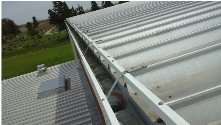
Photo showing condition of the gutter edge. Gutter is flush with metal roof which could cause issues with overflow.
