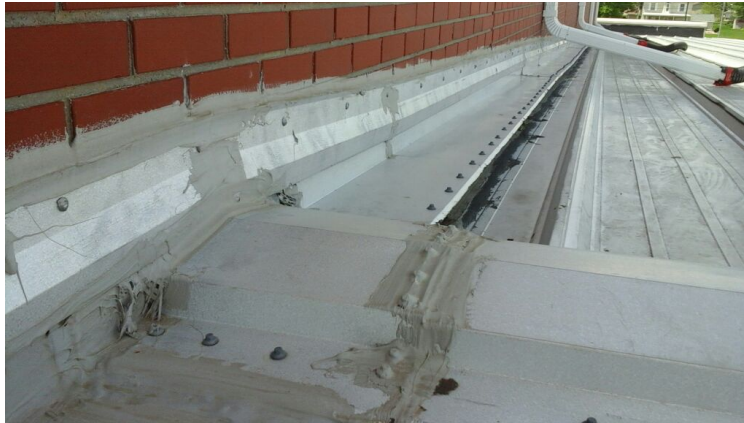
Photo showing condition of the perimeter flashings. Excess caulking has covered top of perimeter flashings.
