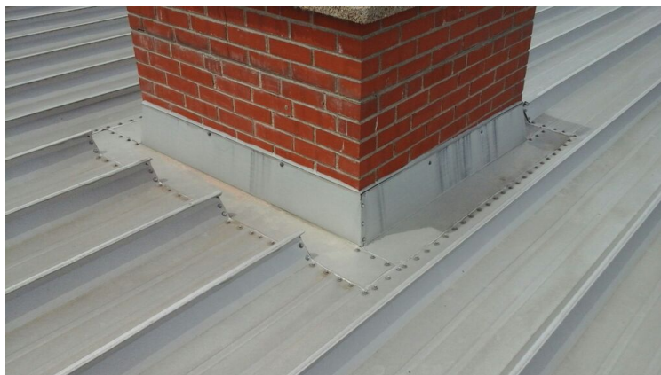
Photo showing condition of projection flashings.
