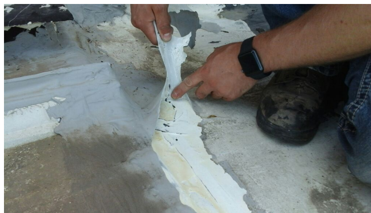
Photo showing caulking pulling up easily. This material is not watertight and is most likely trapping water.
