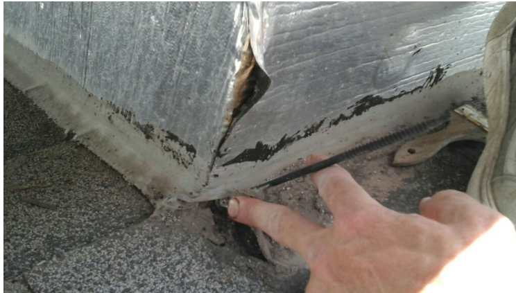
Photo showing projection flashing with a nail and duct tape that was just caulked over.
