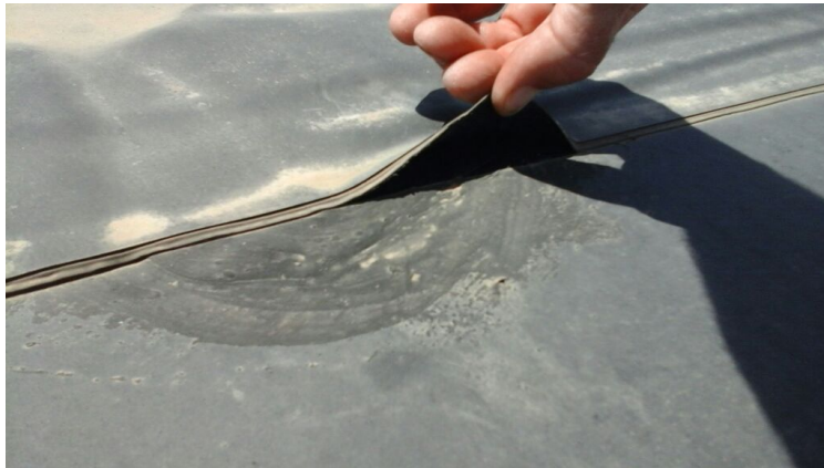
Photo showing strip applied over caulking that is pulling up because it is not adhered properly.
