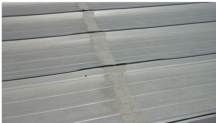
Horizontal seams have been caulked which tends to trap water and pull it through the roof as it deteriorates.
