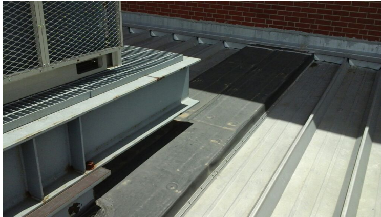
Photo showing flute fill above HVAC units.
