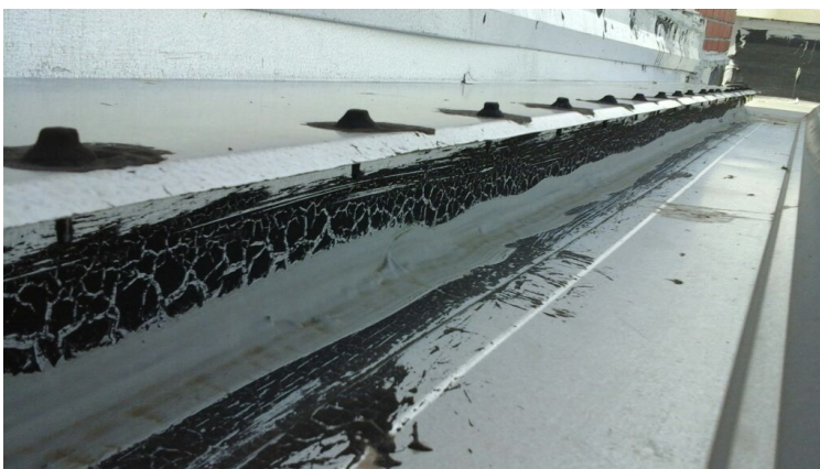
Caulking over tar that pulls right up meaning it is not water tight. This is an area with a leak potentially caused by caulking trapping water where it has failed.
