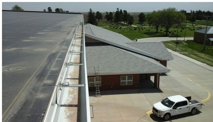
Photo showing condition of the gutter edge.
