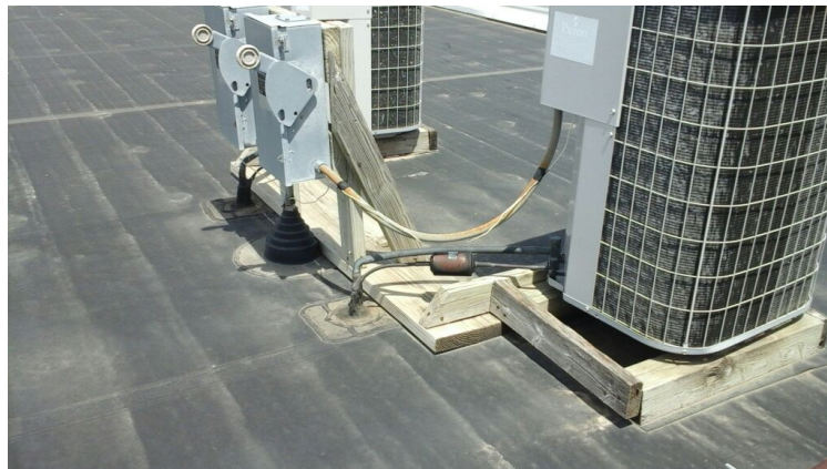
Photo showing condition of sleepers and conduit penetrations.
