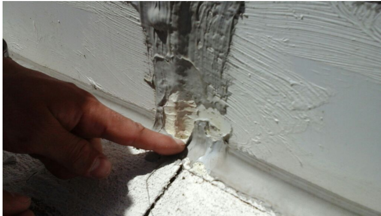
Photo showing caulking on top of caulking in problem leak area.
