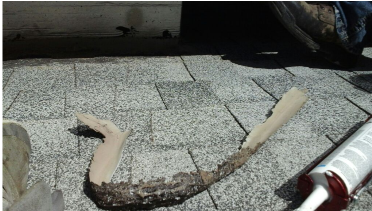
More ineffective caulking that was placed on top of existing caulking. Pulled right up and was doing nothing to prevent water from getting through.
