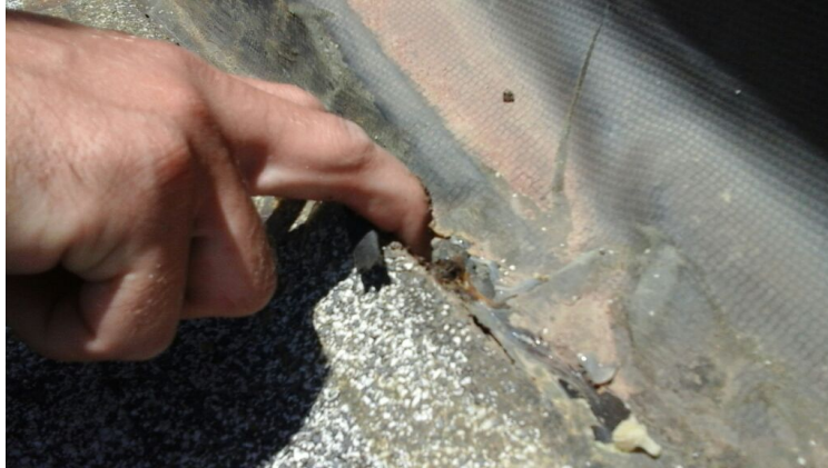
Photo showing another unsealed gap next to roof hatch.
