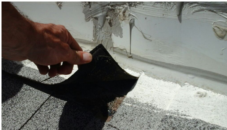
Photo showing shingles on top of flashing pulling loose.
