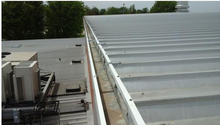
Photo showing condition of the gutter edge.
