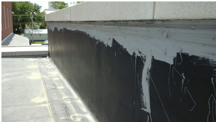
Photo showing ineffective caulking on every joint.
