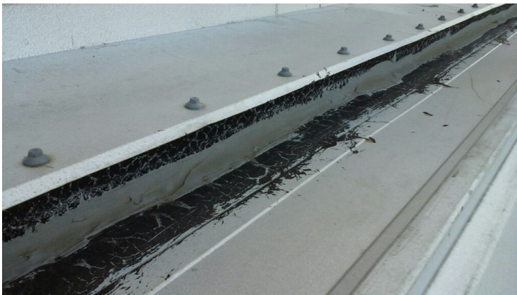
Caulking over the top of tar along the gym wall perimeter.
