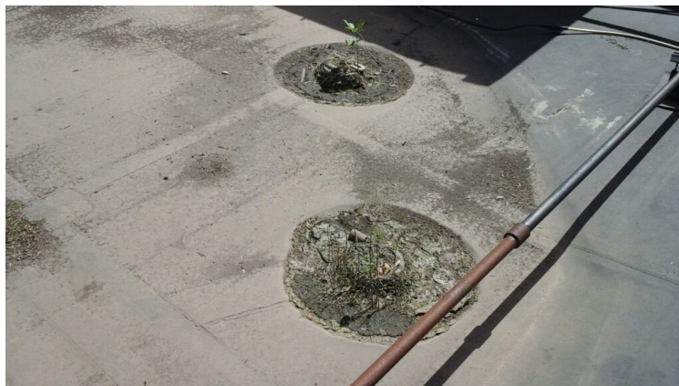
Photo showing drains clogged with debris over where a leak has been occurring. Cleaned out as part of the maintenance agreement.
