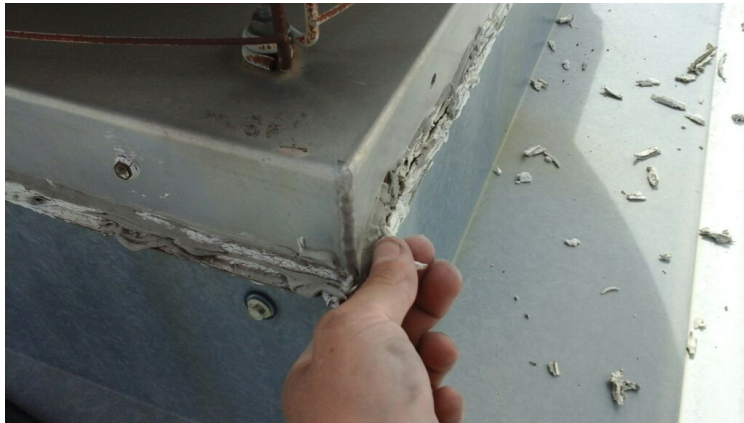
Photo showing projection with undersized metal flashing that was patched with multiple layers of caulking. Repaired as part of the maintenance agreement.
