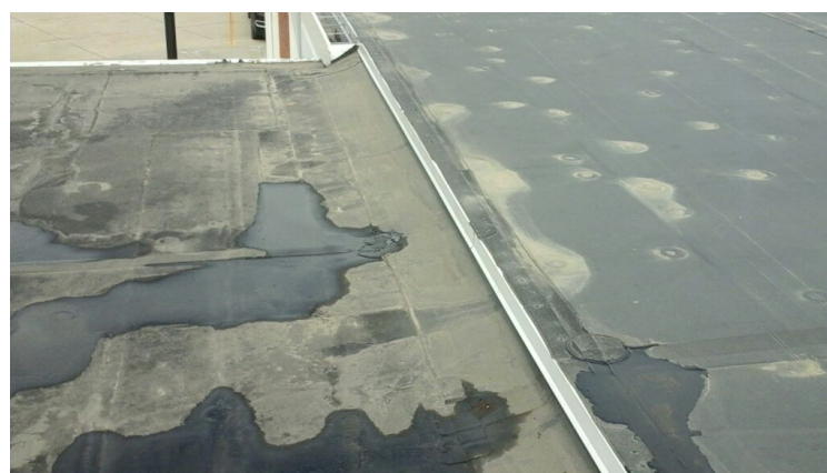
Photo showing delamination along expansion joint.
