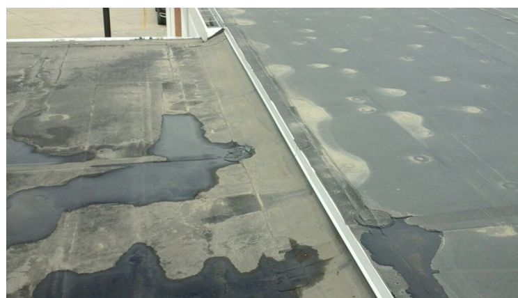
Photo showing delamination along expansion joint.
