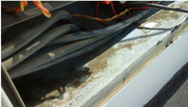
Photo showing visible water stains around holes that lead directly into the office. Repaired as part of the maintenance agreement.
