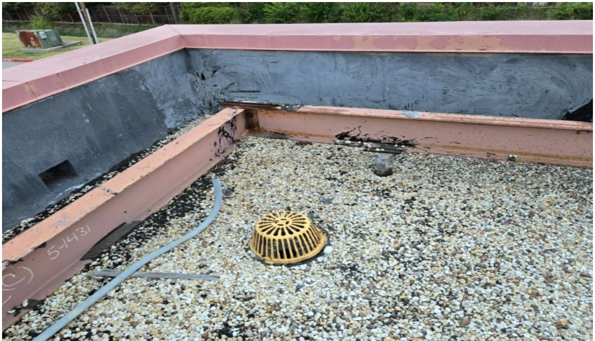
Old gravel will be removed and any pipes will be raised and lifted off the new roof system.
