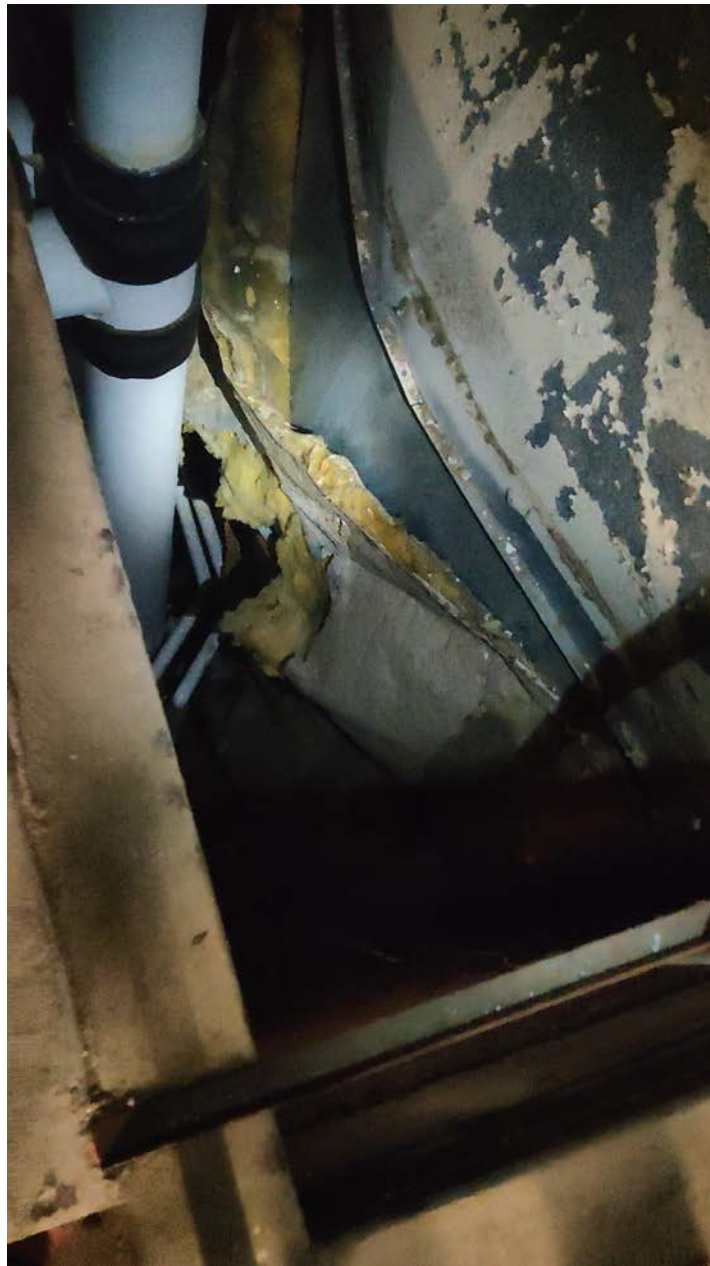
Figure 2. Large visible penetration in the duct of AHU-D2
