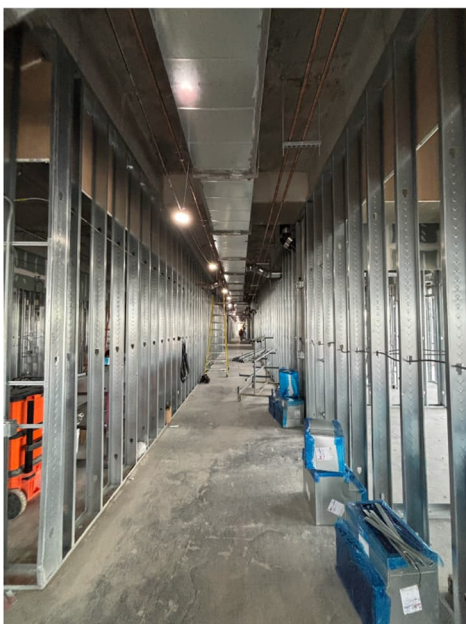
Main Corridor with HVAC Duct, Plumbing Lines, and Medical Gas Lines
