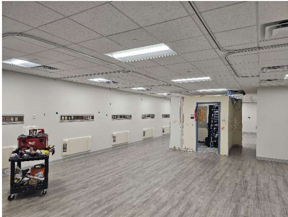
1st Floor LVN Lan with Old IDF Closet
