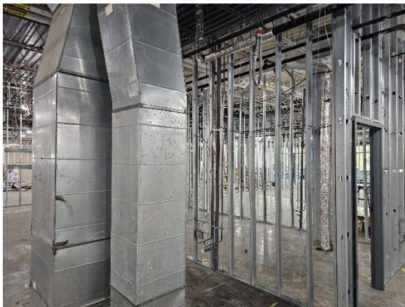
Science Labs Duct Work
