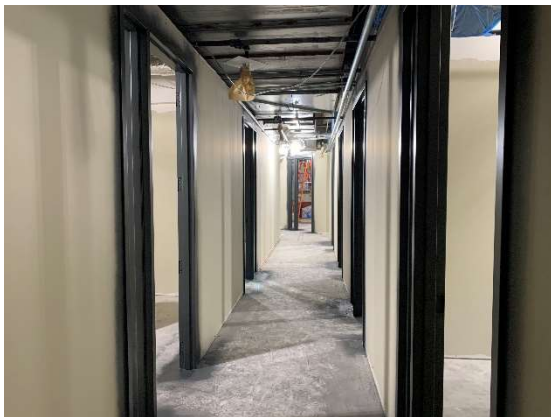
Door Frames at Dental Offices
