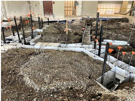
Void Boxed Plumbing in Kitchen Area
