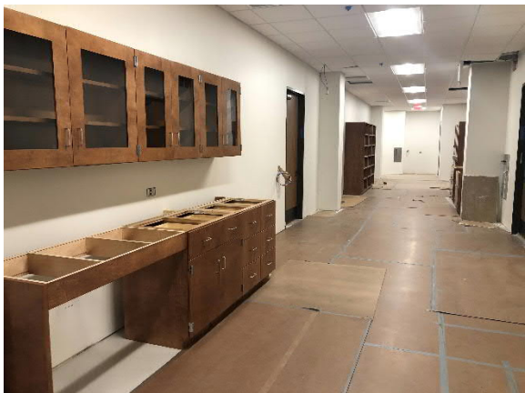
Casework Installed in Campus Commons Lab Space
