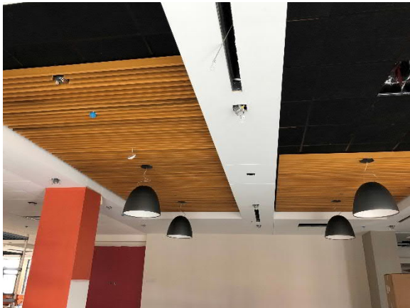
Wood Ceiling and Light Pendants Installed in Lounge Area of Student Center
