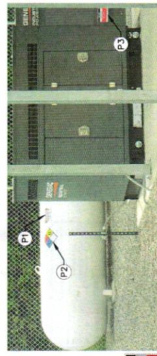
FIGURE 7 - PROPANE TANK & GENERATOR SIGNAGE
