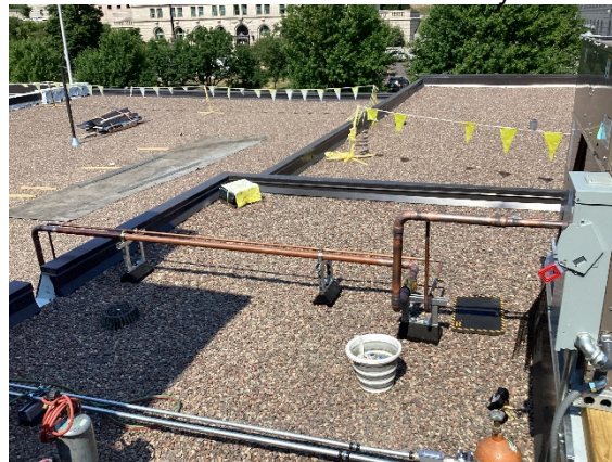
HVAC/ Plumbing Systems on Roof
