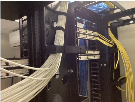
Data Rack and Cabling
