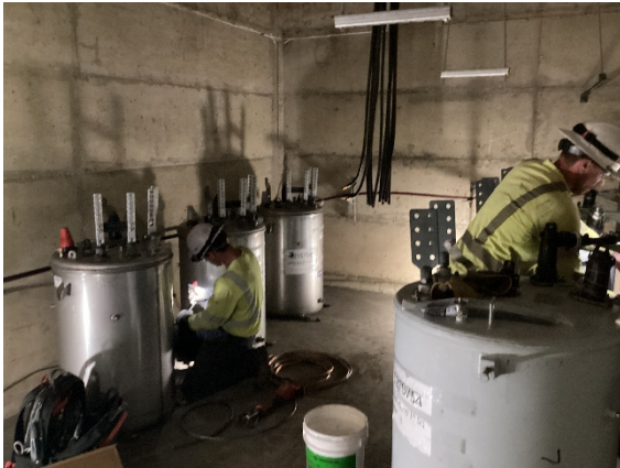
New Electrical Service
