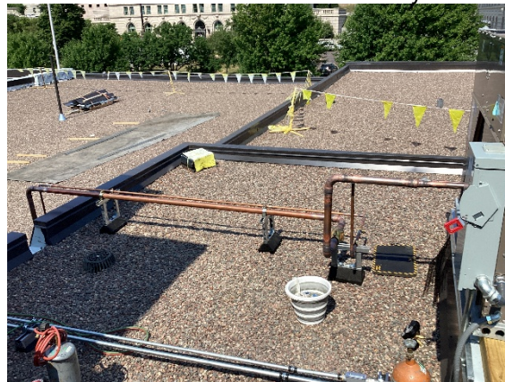
HVAC/ Plumbing Systems on Roof
