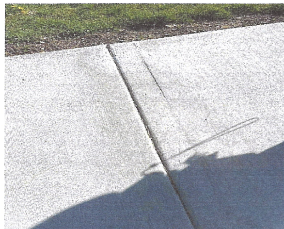
Fig. 2 - Uneven Control Joint
