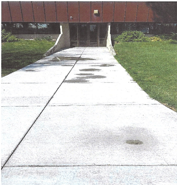
Fig. 9 – Water ponding – improper pitch
