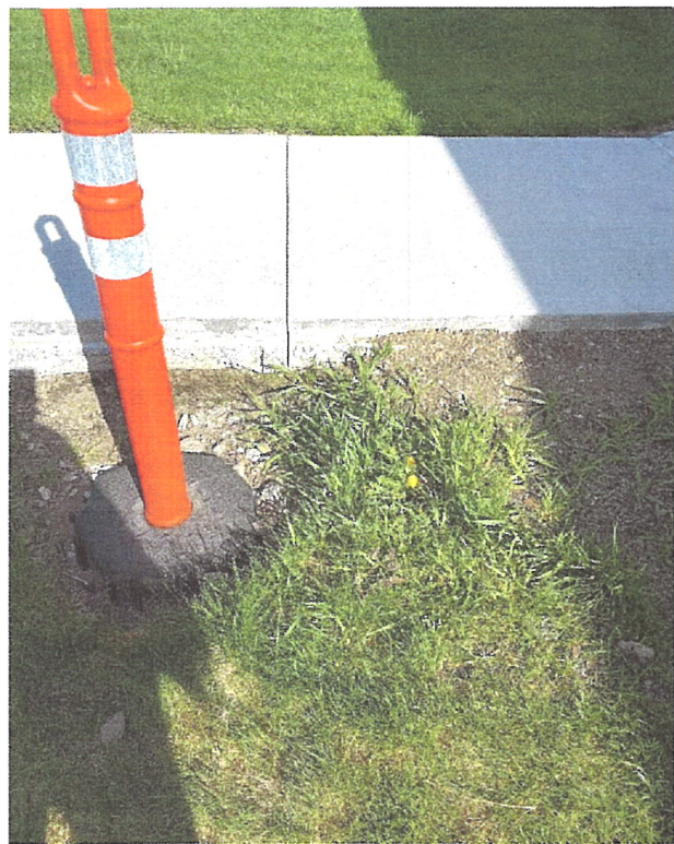
Fig. 8 – Incomplete edge restoration
