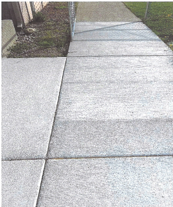
Fig. 3 – Uneven Broom Finish
