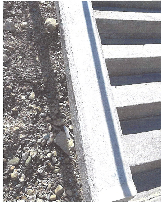
Fig. 12 – Defective surface finish
