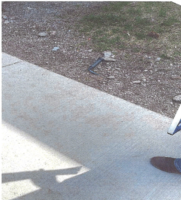
Fig. 5 – Incomplete irrigation restoration
