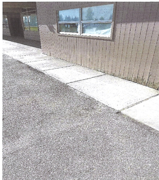
Fig. 10 – Incorrect asphalt patching
