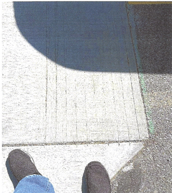
Fig. 6 – Defective detectable warning grooves
