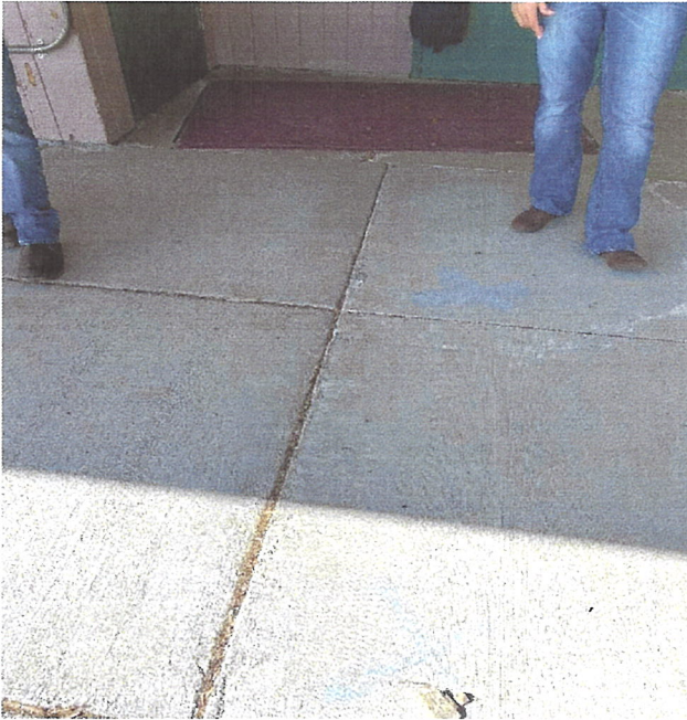
Fig. 11 – Missing expansion joint
