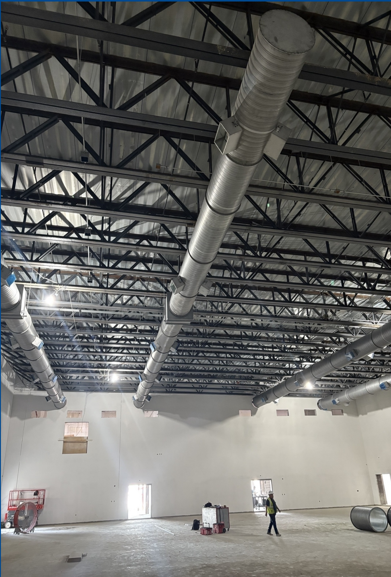
Gym/Storm Shelter Duct
