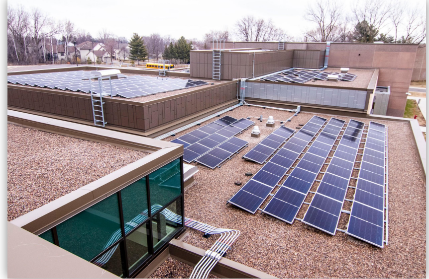
Eagle Point Elementary - 3,930 kW array
