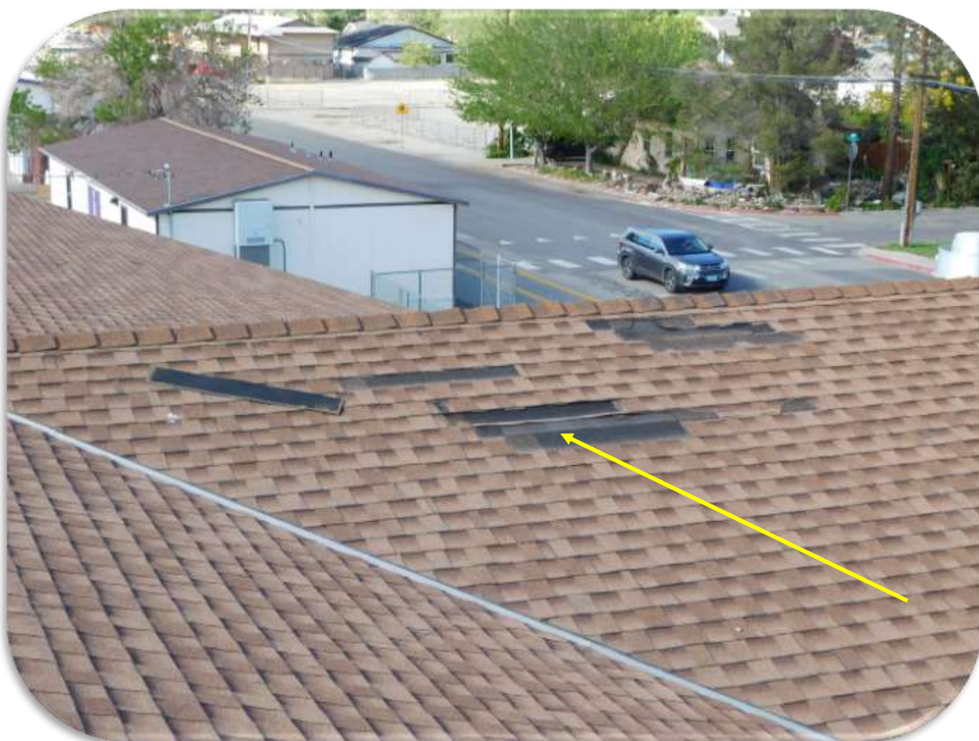
OVERVIEW OF THE EAST WING BUILDING = MPR SHINGLES MISSING AT THIS AND ANOTHER LOCAL.
