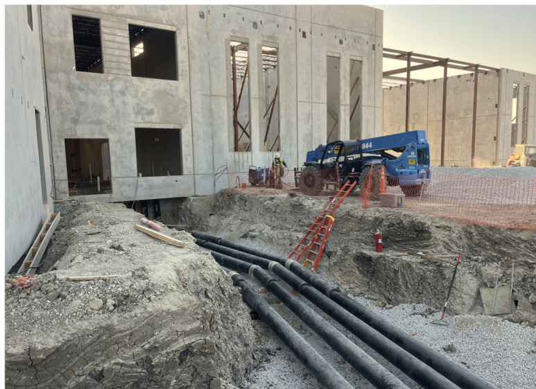
Hydronic Piping Entering the Building
