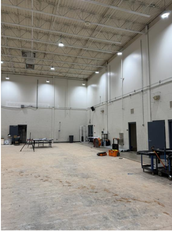
POM_CHEER BUILDING OVERHEAD ELECTRICAL
